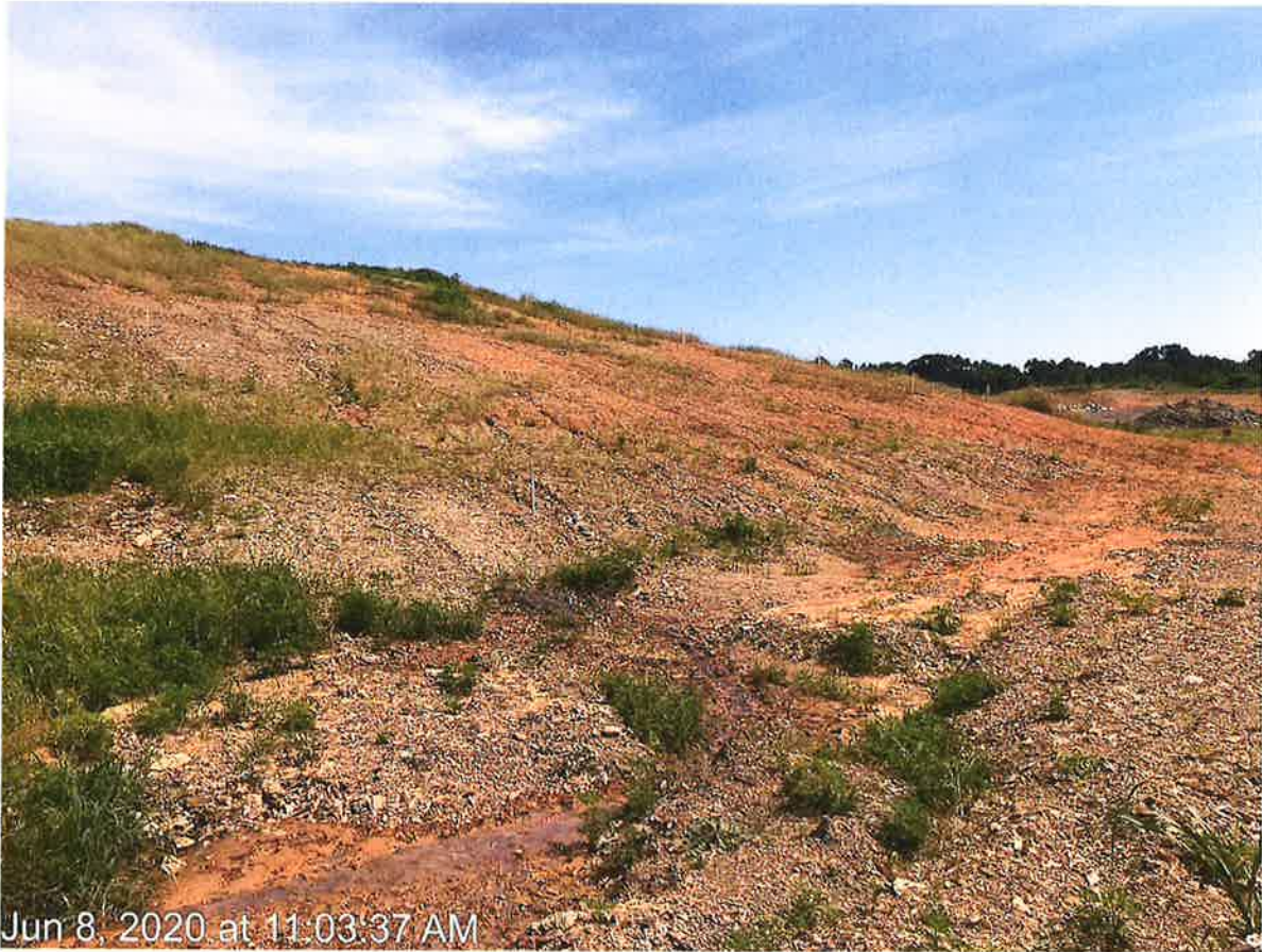
Figure 4 - Leachate outbreak and stream on southeast facing slope
