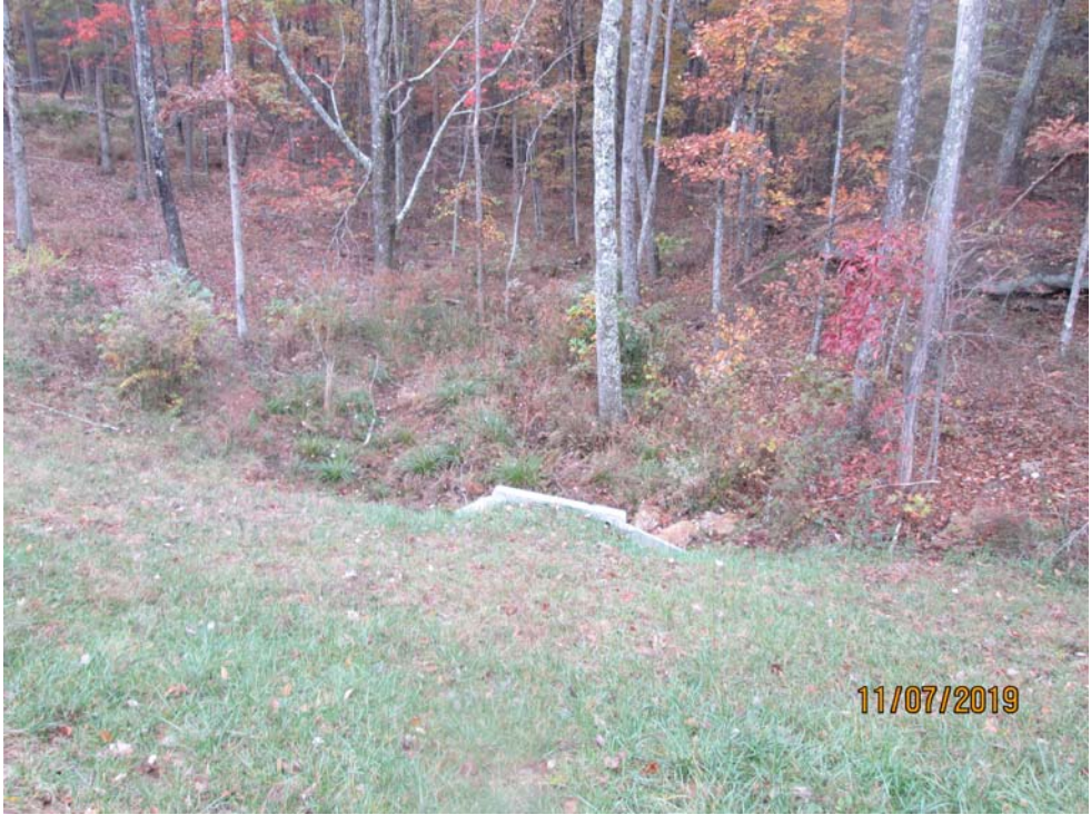
Photo 4: Minor Road Crossing #2 View of the stabilized upstream end of the road crossing. Photo Taken 11/7/2019
