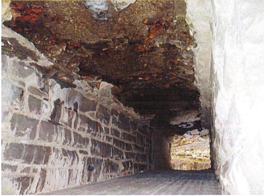
View of undermined culvert floor, north barrel
