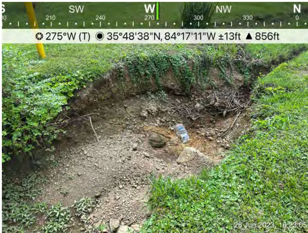
Photo 4 – Location of exposed pipe. Pipe is exposed and gets recovered by periodic high flows.
