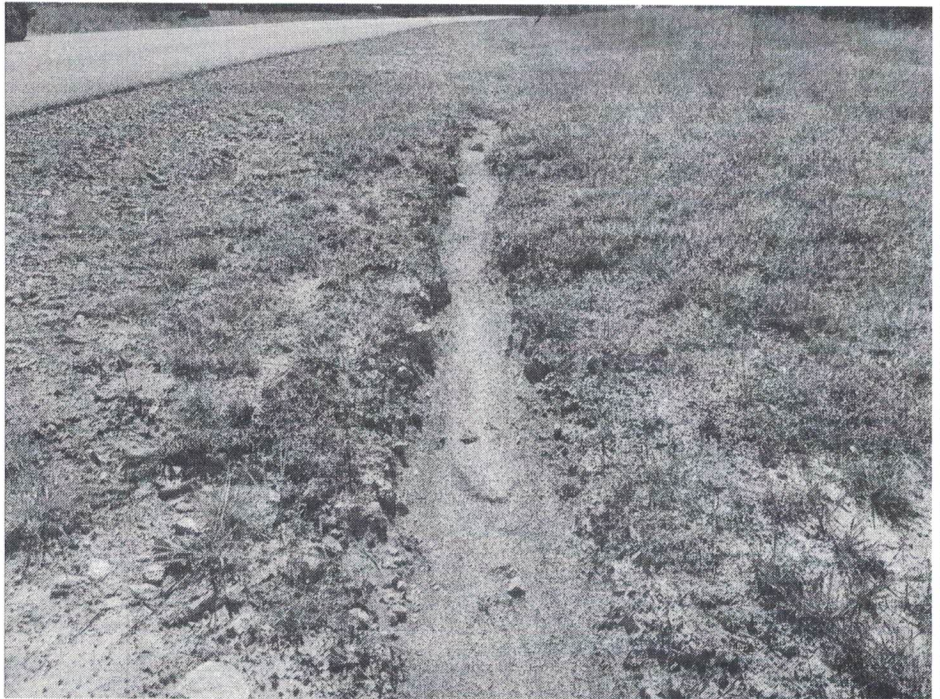
Photo 5: Outfall S201 A roadside swale was observed. The swale should be stabilized with grass, matting, rock, or other means to prevent washout. Check dams may be needed to capture sediment until the swale is stabilized. Photo Taken 8/31/2023
