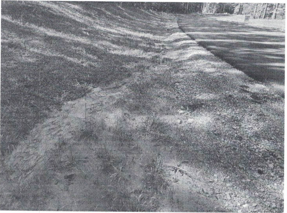
Photo 8: Outfall S275 Areas recently disturbed for utility installation should be stabilized. Rock check dams may be needed in roadside swales to control sediment. Photo Taken 8/31/2023
