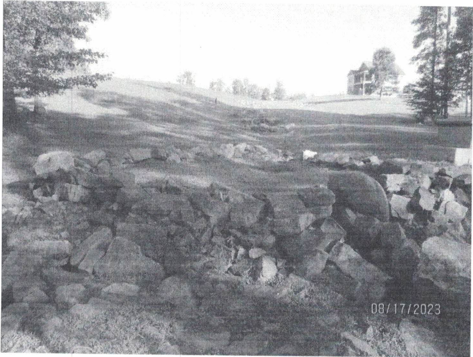
Photo 3: Outfall S98 Rock check dams have been installed in a roadside ditch and appear to be functioning properly. Photo Taken 8/17/2023
