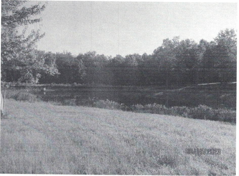
Photo 4: Outfall S153 A stormwater basin has been installed and appears to be functioning properly. Photo Taken 8/17/2023
