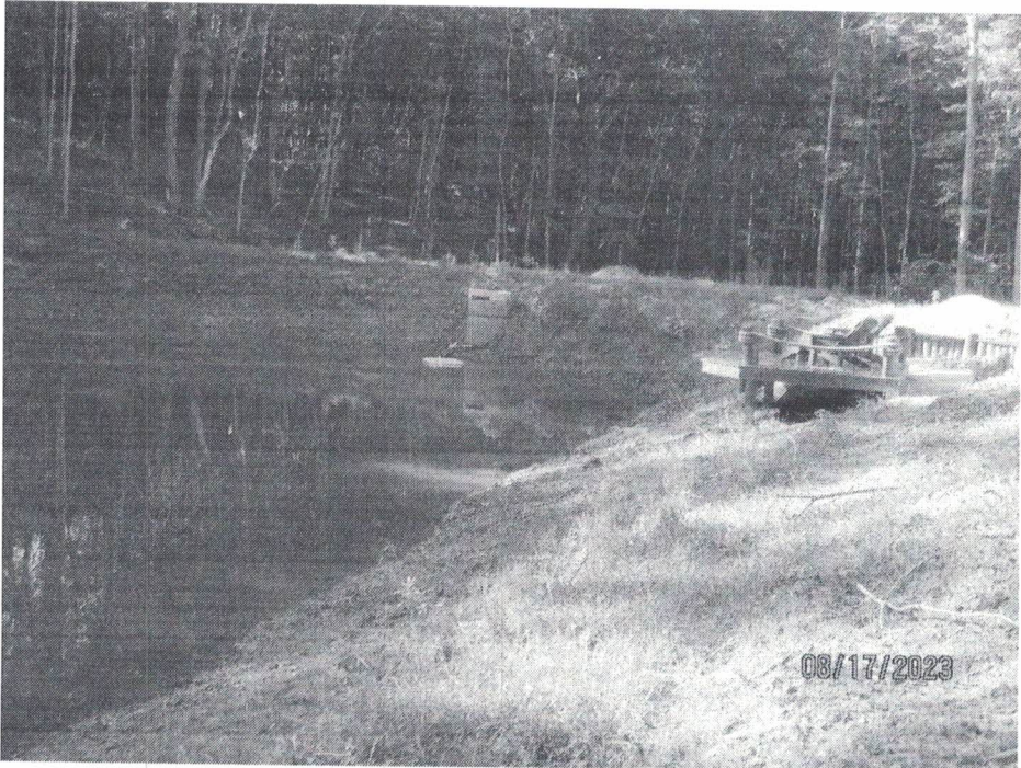
Photo 7: Outfall S218 A stormwater basin has been installed and appears to be functioning properly. Photo Taken 8/17/2023
