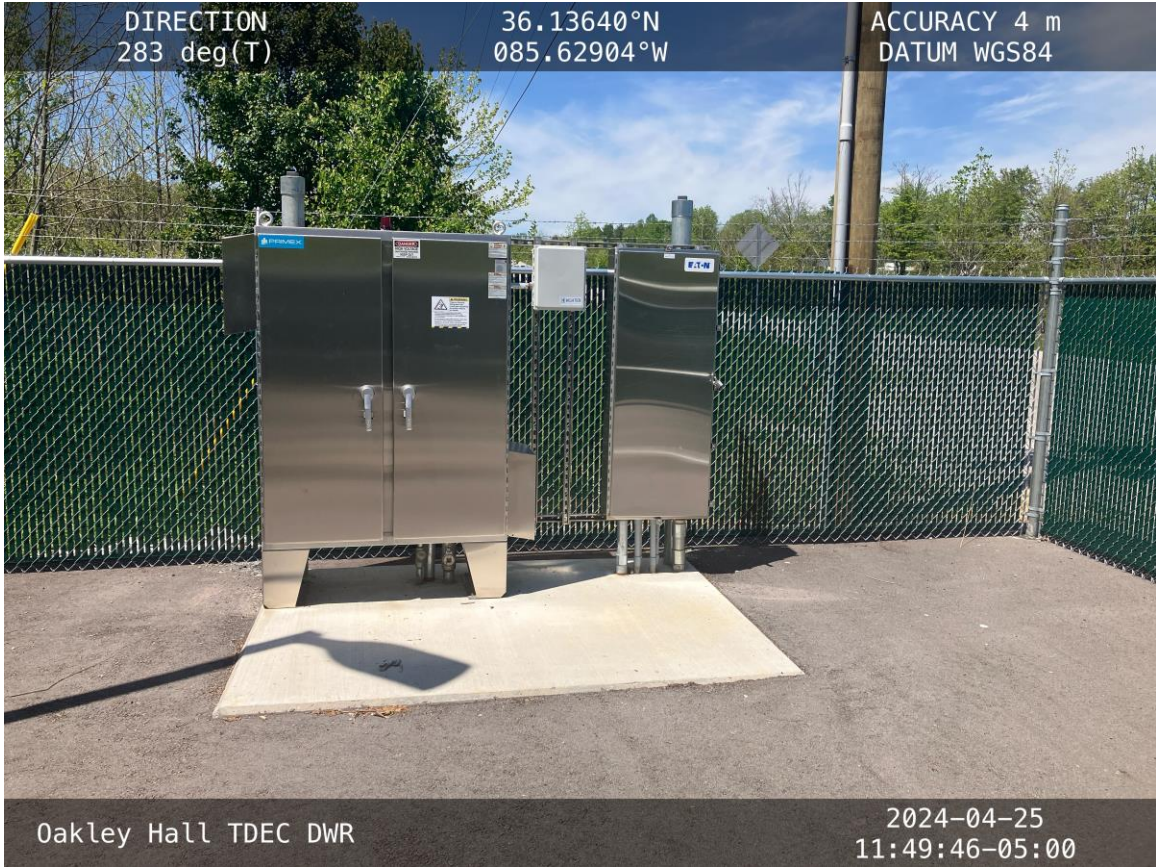
Two new lift stations were visited during the inspection. This one is located adjacent to I-40, on the south side. Note the green slats woven in the chain-link fence.
