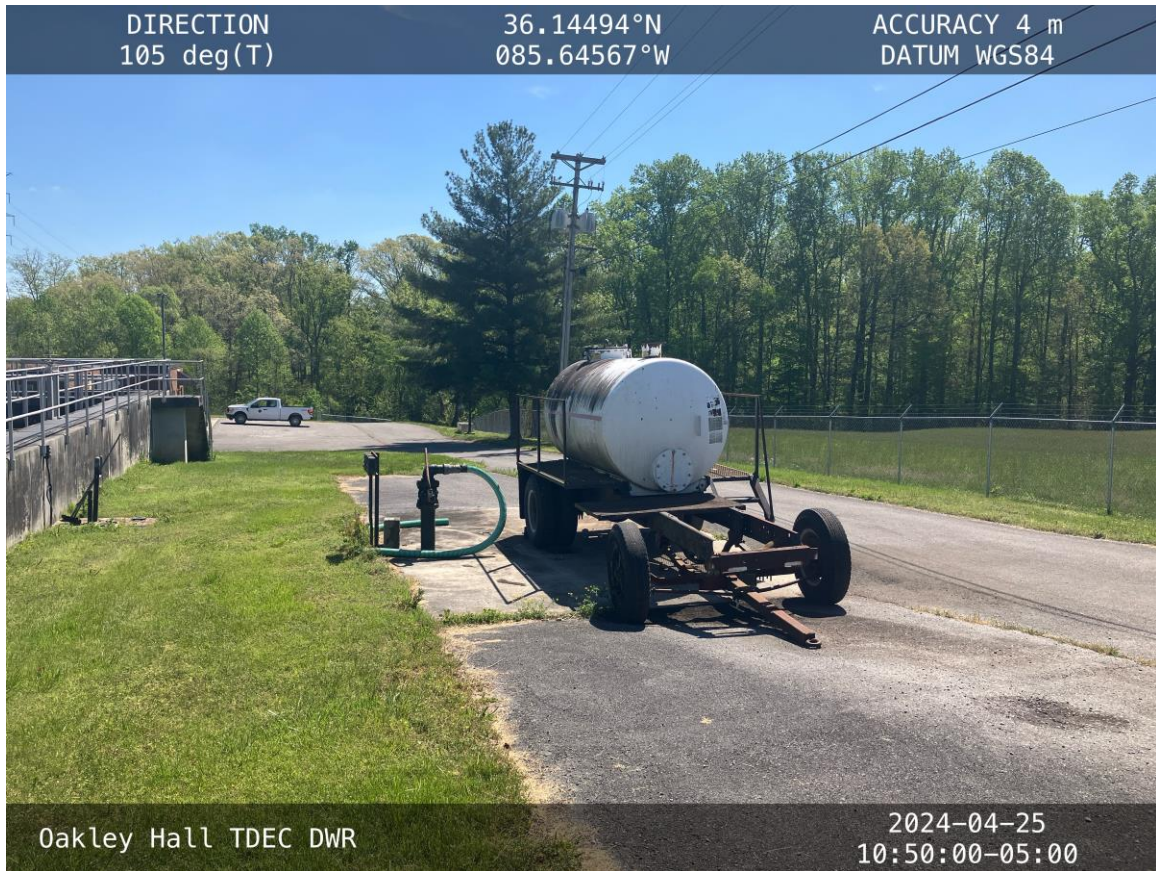
The grounds were clean and well maintained. A tractor is used to pull this liquid biosolids trailer across the surface of an adjacent field. Mechanical problems have recently occurred with the trailer and have been corrected. Photo By: Oakley Hall, April 25, 2024
