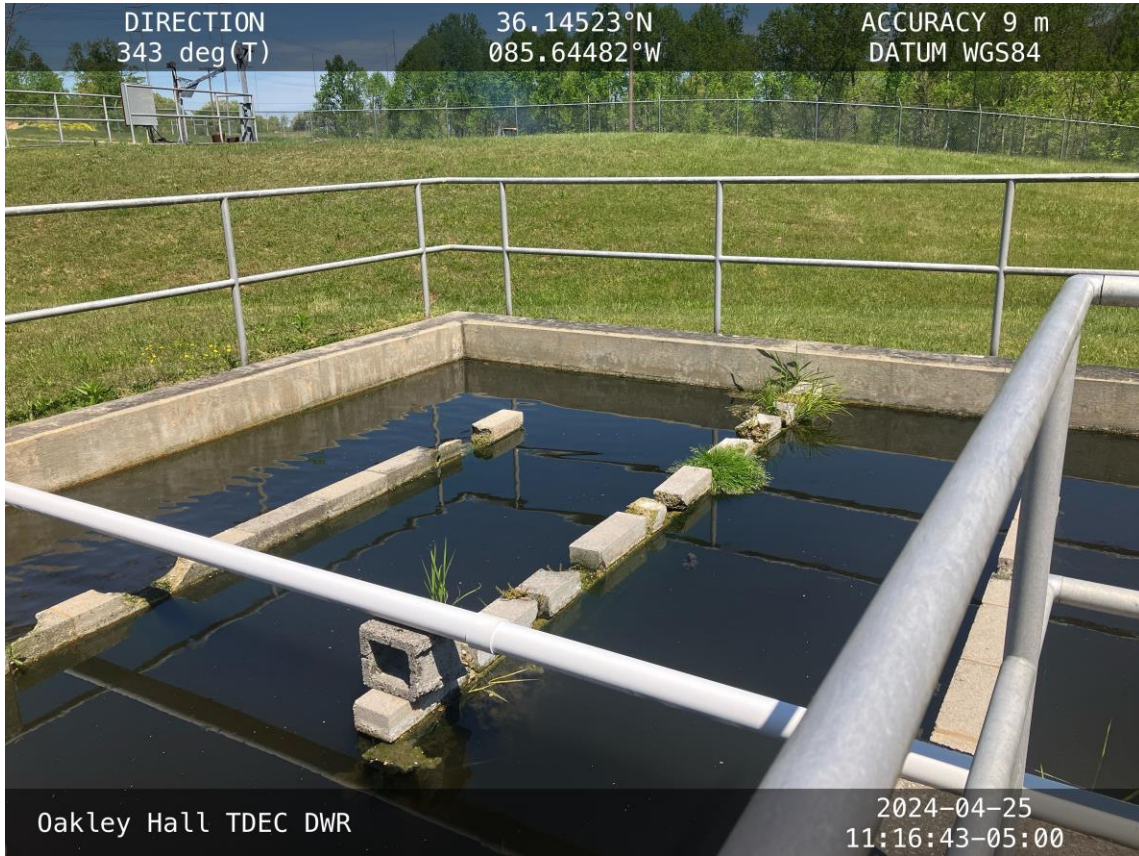
The Chlorine Contact Chamber is pictured. The chamber needs some block work improvements, to reduce short circuiting across the surface. Photo By: Oakley Hall, April 25, 2024
