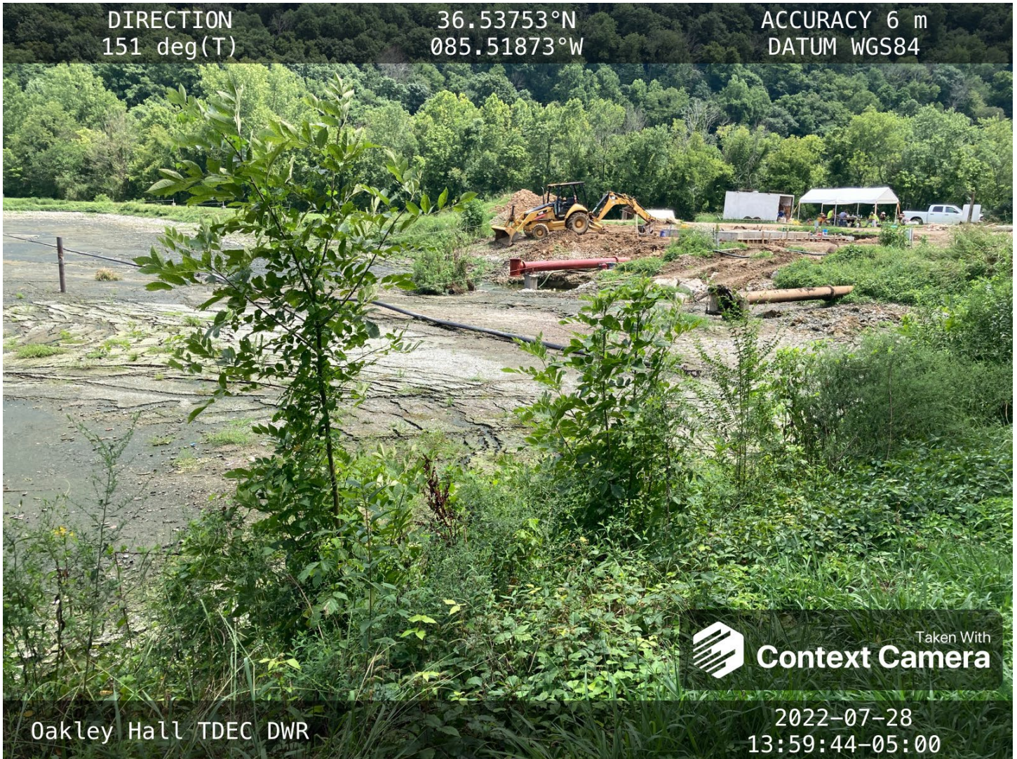
The construction area of the new headworks is pictured. Note the heavy solids in the first treatment pond.
