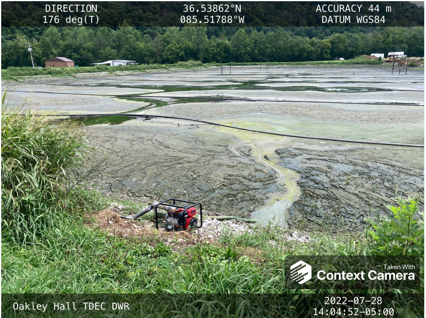
Two pumps are being used to assist draining the first pond as it is bypassed.
