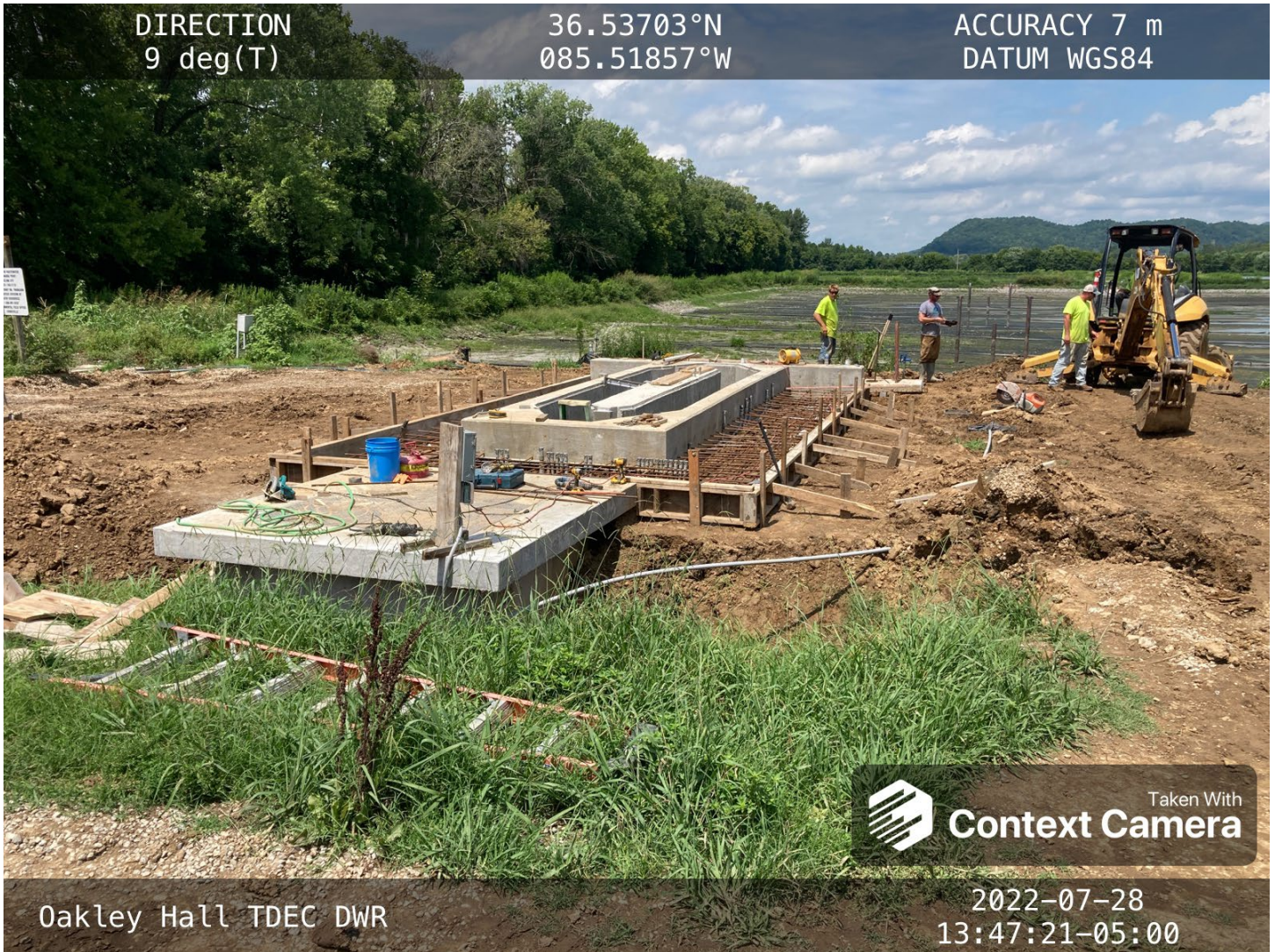
The third iteration in headworks is being constructed for this sewer treatment system.
