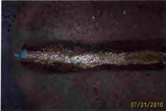
Downstream sewer from O'Charleys- Moderate FOG.
