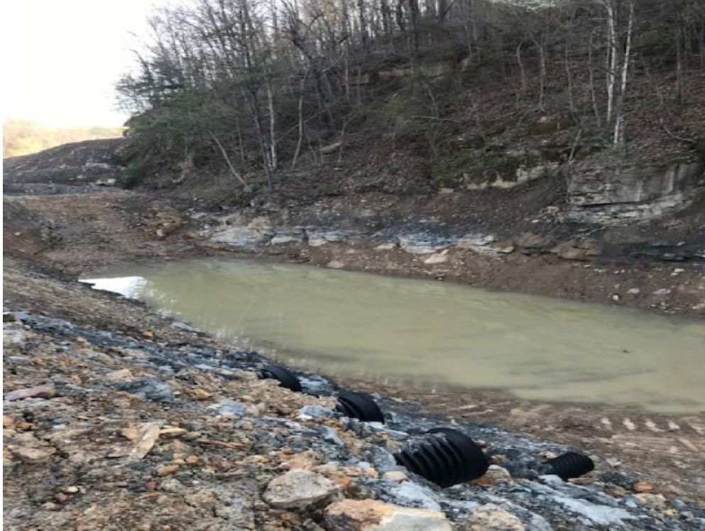
Pic 4 Pond 100 Sealed and Auger Holes Plugged (above white rock line in back)
