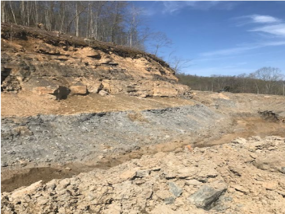
Pic 9 Pond 103 during construction and sealed auger holes above gray shale line
