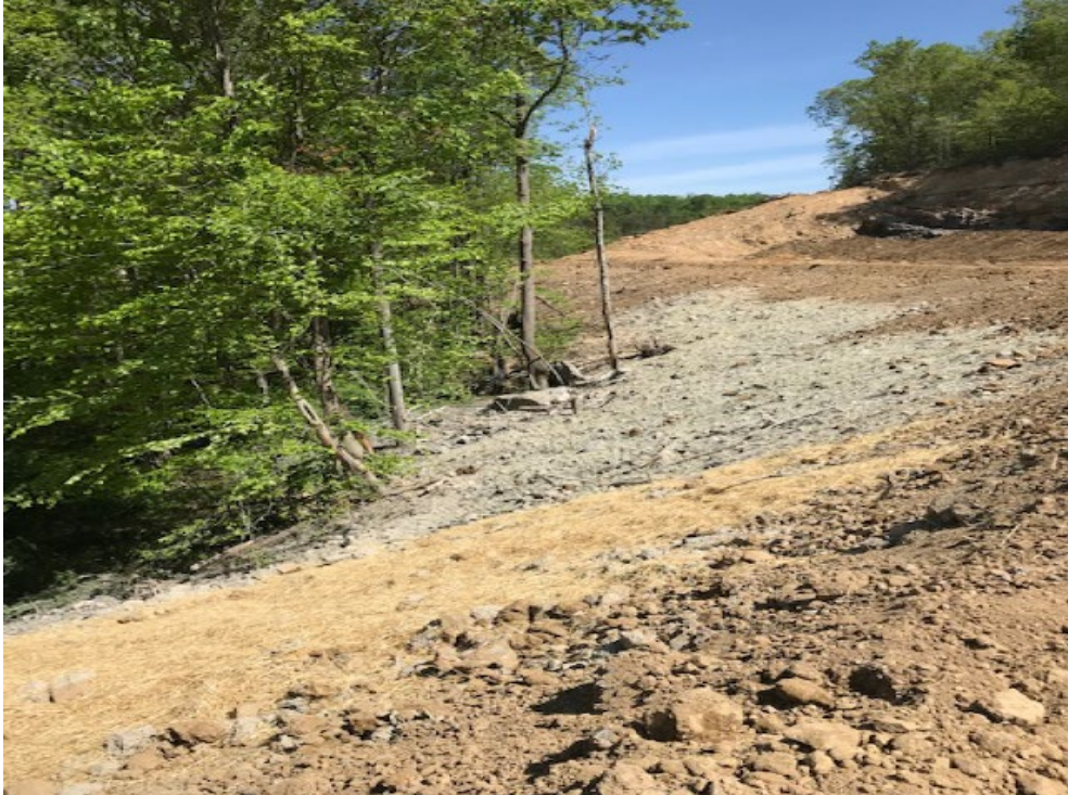
Pic 16 Berm, ditch, timber separated with one spot left to seed near very end of job (5-5-22)
