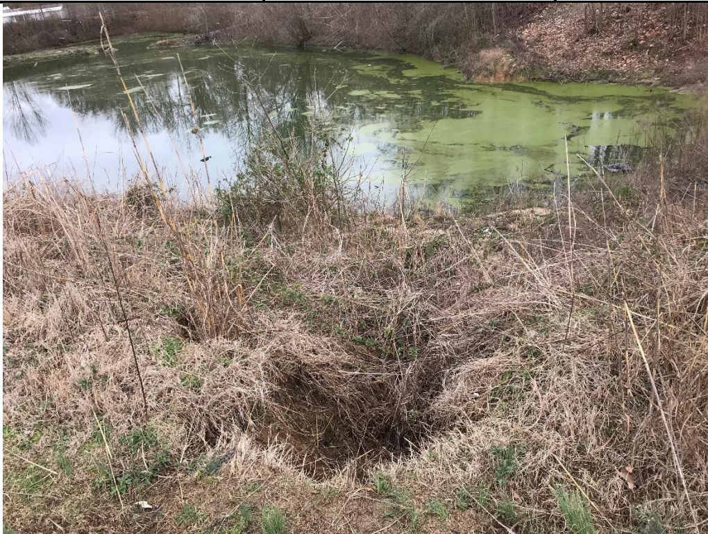
Photo 8. View of an eroded area on the northern portion of the wastewater treatment lagoon.
