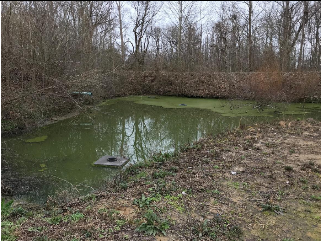
Photo 2. View of the southern portion of the wastewater treatment lagoon. The aerator serving the southern portion of the lagoon was inoperable during the inspection.
