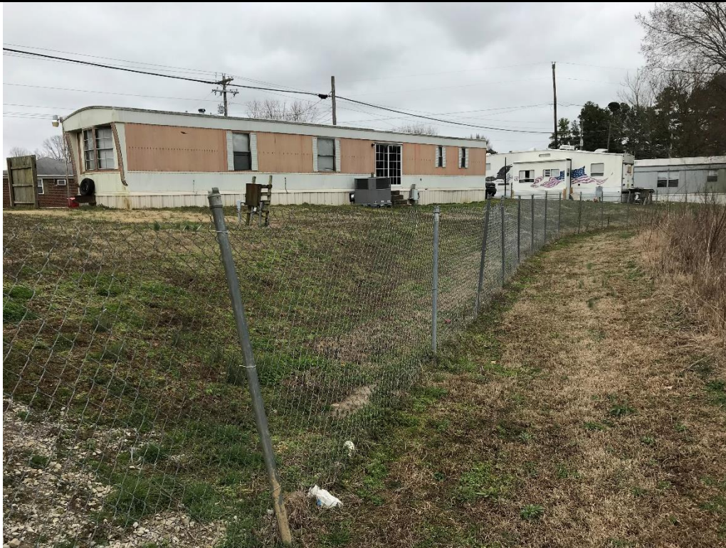
Photo 7. Representative example of the chain link fence surrounding the perimeter of the wastewater treatment lagoon. The appropriate signs were not posted at regular intervals (at least every 150 ft.) around the perimeter of the wastewater treatment lagoon.
