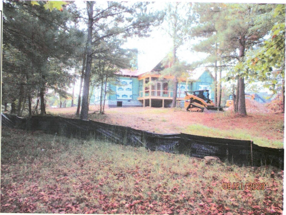
Photo 1: Outfall S59 The individual lot level erosion controls have been installed and appear to be functioning properly. Photo Taken 9/21/2023
