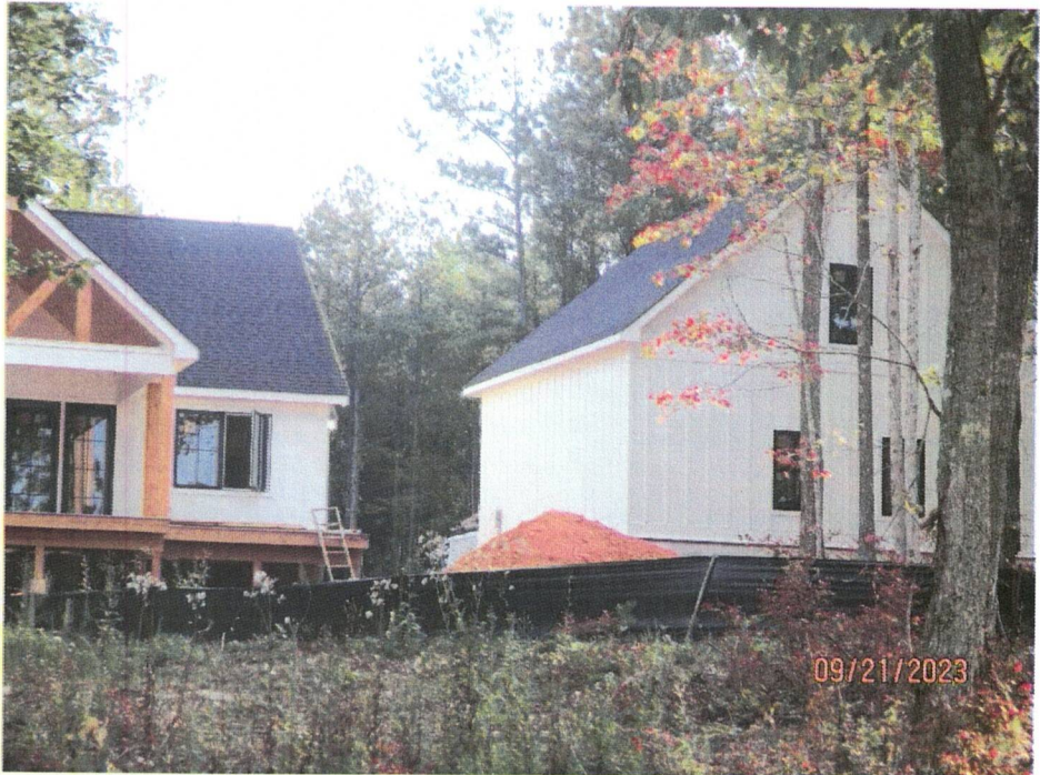
Photo 8: Outfall S275 The individual lot level erosion controls have been installed and appear to be functioning properly. Photo Taken 9/21/2023
