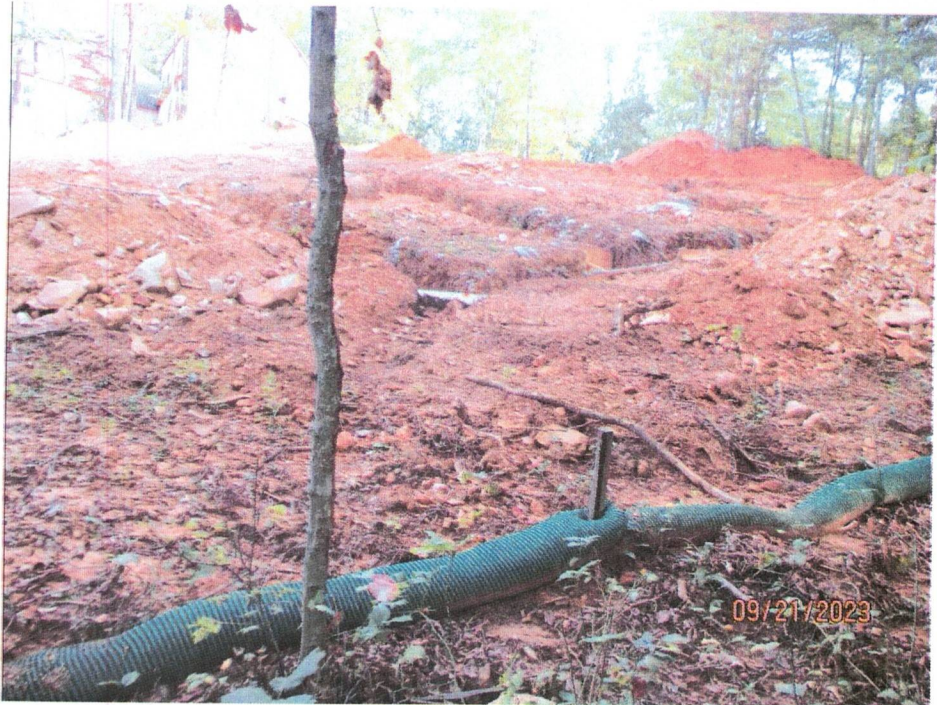
Photo 7: Outfall S218 The individual lot level erosion controls have been installed and appear to be functioning properly. Photo Taken 9/21/2023
