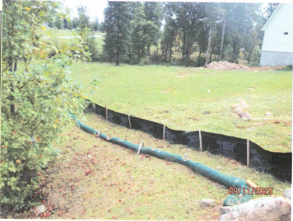
Photo 1: Outfall S59 The individual lot level erosion controls have been installed and appear to be functioning properly. Photo Taken 9/11/2023
