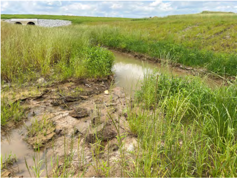
22 Stream 1-A Diversion confluence with Stream 9, facing downstream and to the northeast
