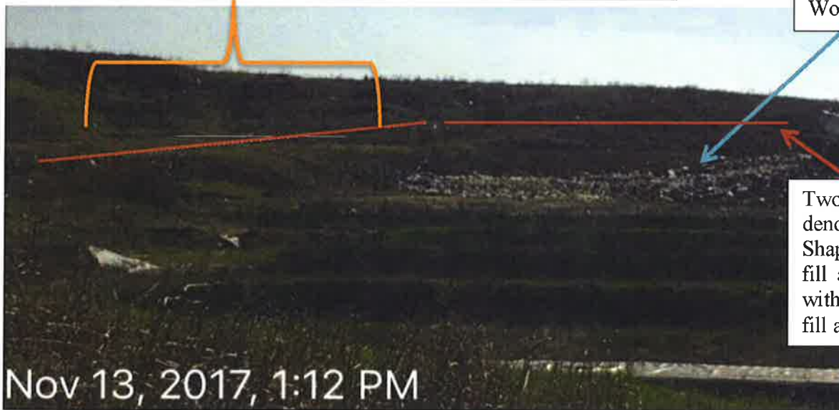
Picture 3. The City of Dyersburg Landfill inspection on November 13, 2017: Photo of repaired inner slopes that were observed with erosion, washout of solid waste, unsatisfactory intermediate cover, and unsatisfactory stabilization of cover on the October 27, 2017 inspection.
