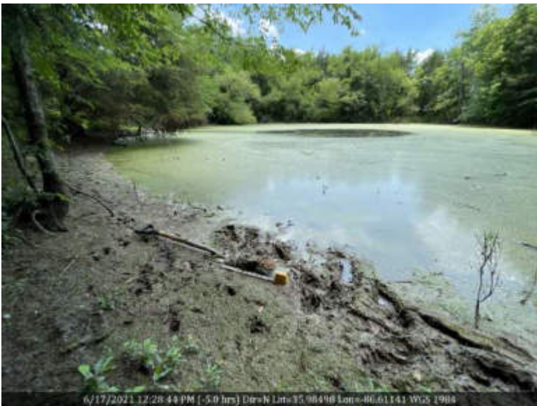
27 View of upper, northern end of ISOPND-A and soil profile with clay liner, facing south.
