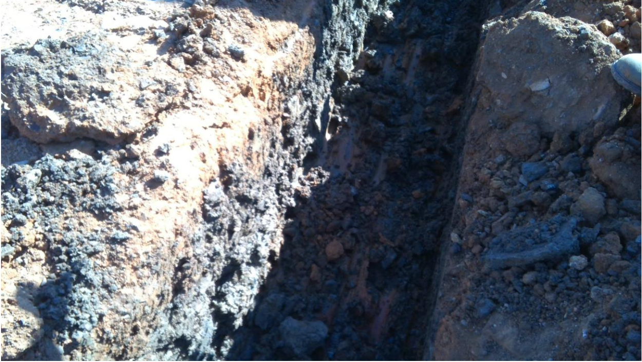
Photo 1: Typical Bottom of Connection Trench with Clay Liner Exposed and Protective Shale Layer along the Trench Walls
