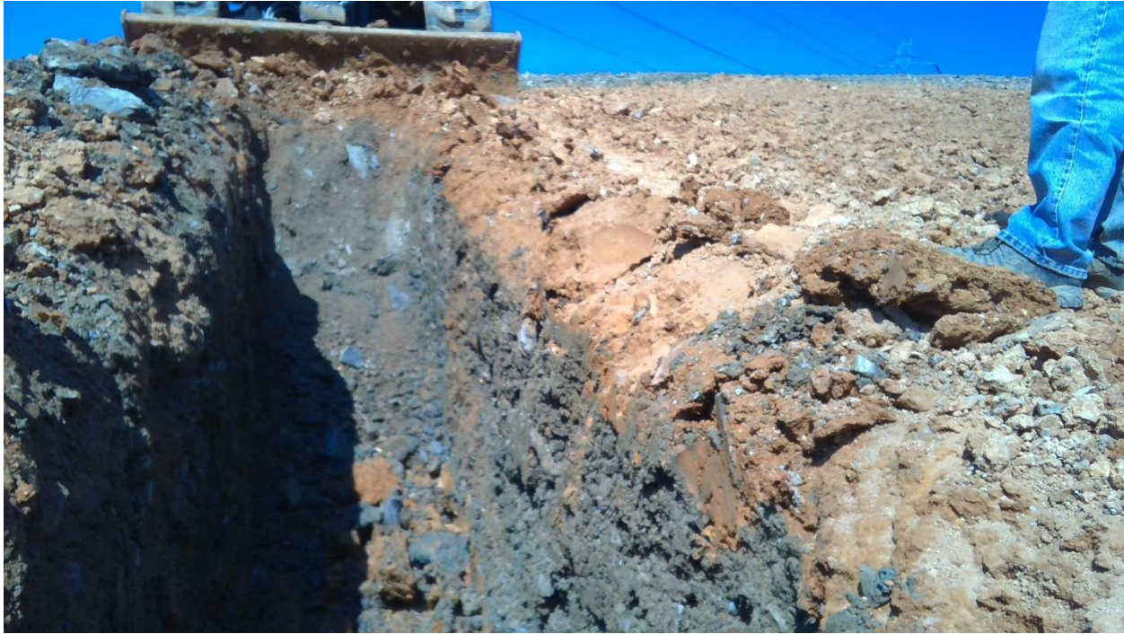
Photo 5: Western Extent of Connection Trench at the Edge of the Clay Liner
