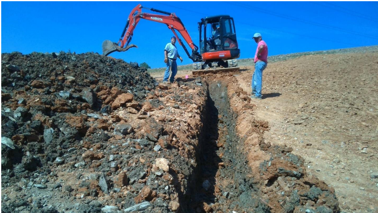
Photo 4: Excavation of Connection Trench West of Drainage Basin inlet for Stormwater Pond 1
