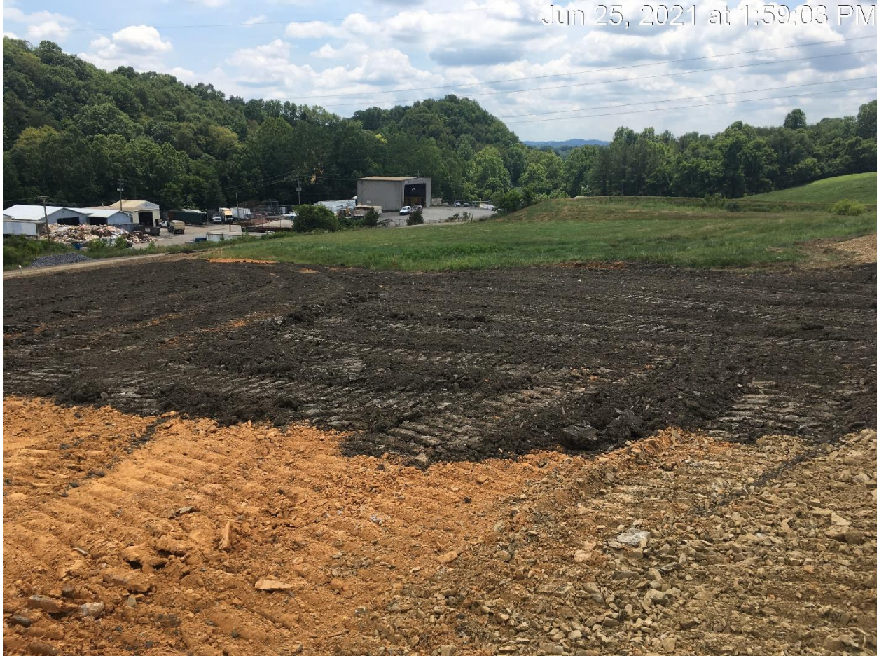
Figure 6: FIRST LIFT OF TOPSOIL BETWEEN THE LOWEST TACK-ON BERM AND THE SECOND TACK-ON BERM
