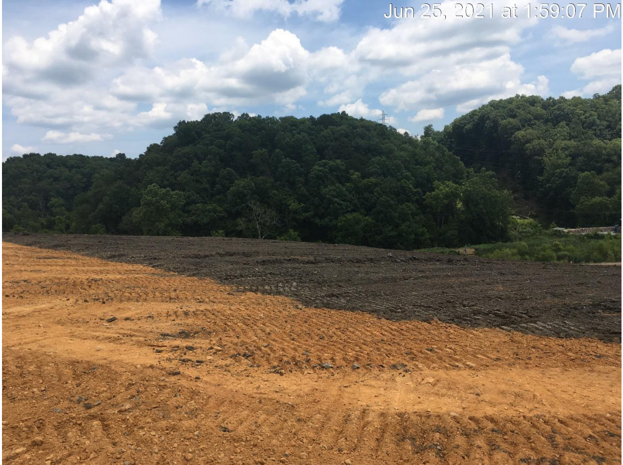
Figure 7: FIRST LIFT OF TOPSOIL BETWEEN THE LOWEST TACK-ON BERM AND THE SECOND TACK-ON BERM
