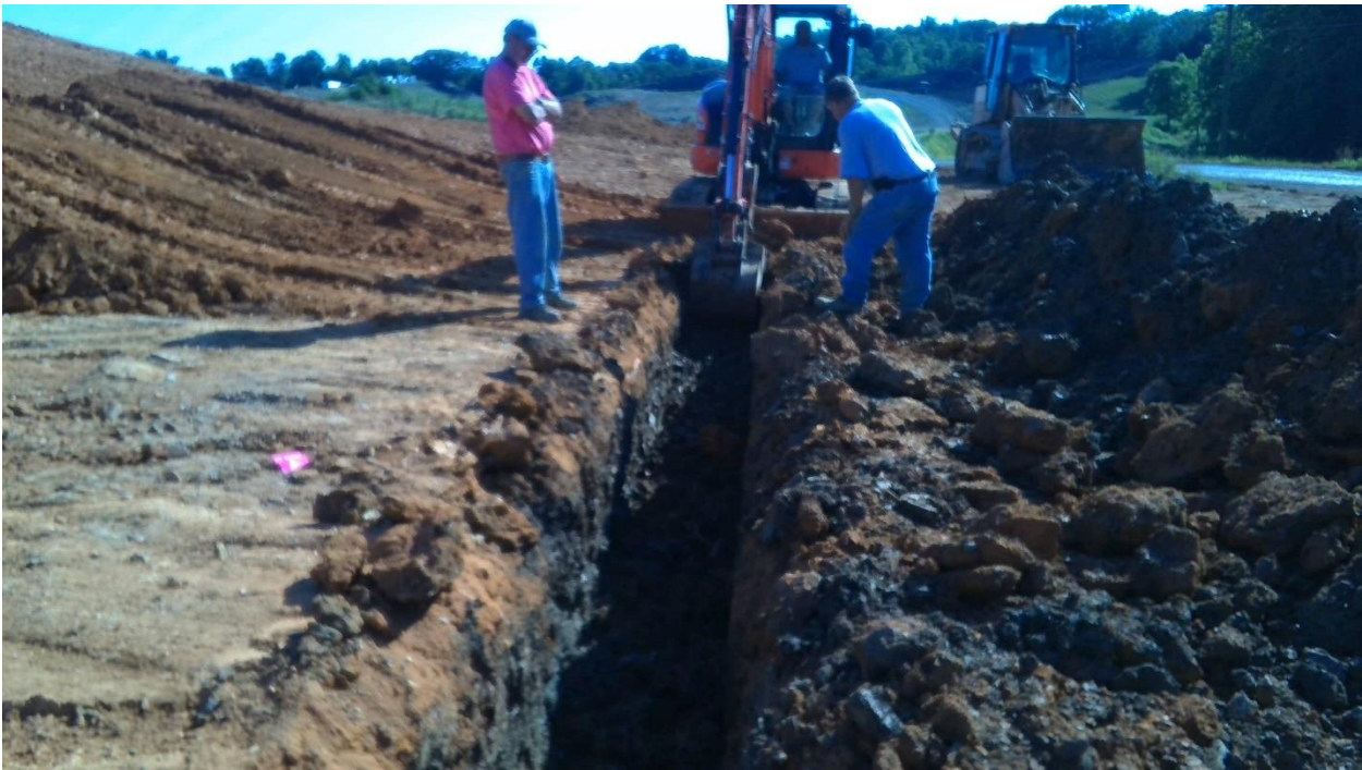
Photo 2: Excavation of the Connection Trench using an Excavator with a Two-Foot Bucket
