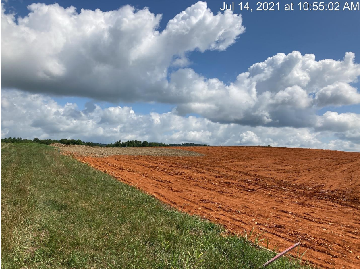
Figure 2: SHALE AREA IN THE NORTH EAST CORNER OF THE CLOSURE AREA
