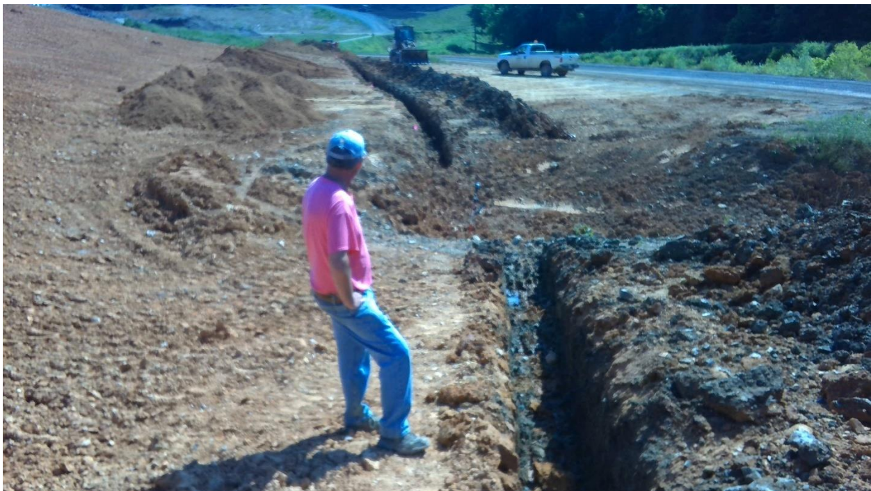
Photo 6: Full Length of Connection Trenches. Gap between Trenches is the Drainage Basin inlet for Stormwater Pond 1. The bottom of the Drainage Basin is approximately four-feet below the observed Clay Liner. Stockpiled Clay for Backfilling the Trench is located to the Left of the Trench.
