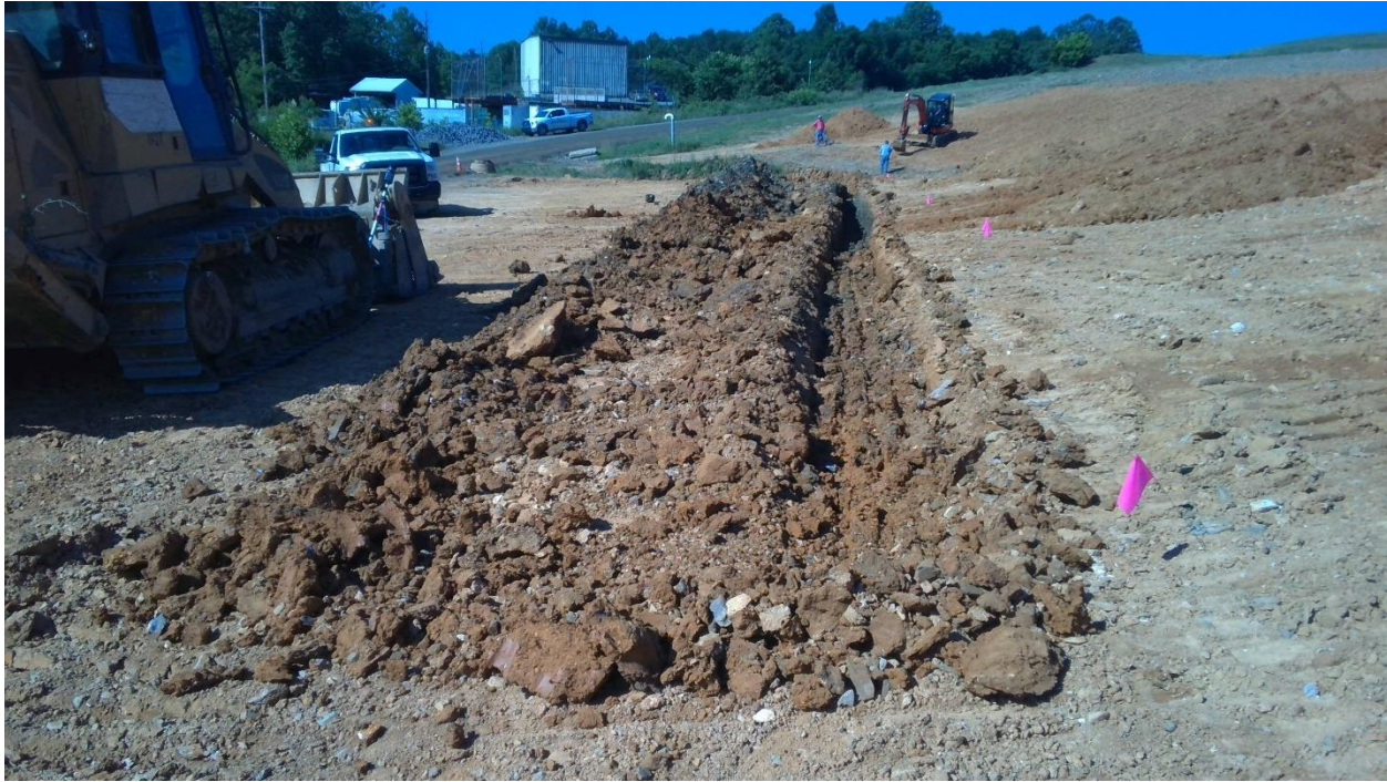
Photo 3: Full Length of Connection Trench East of Drainage Basin inlet for Stormwater Pond 1
