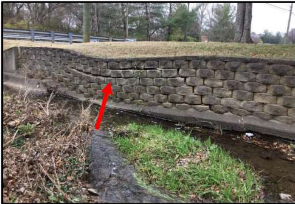
Figure 2 - View of CMU Retaining Wall (Notice bulge in wall)
