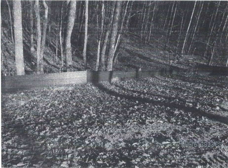
Photo 6: Outfall S218 The individual lot level erosion controls have been installed and appear to be functioning properly. Photo Taken 11/16/2023
