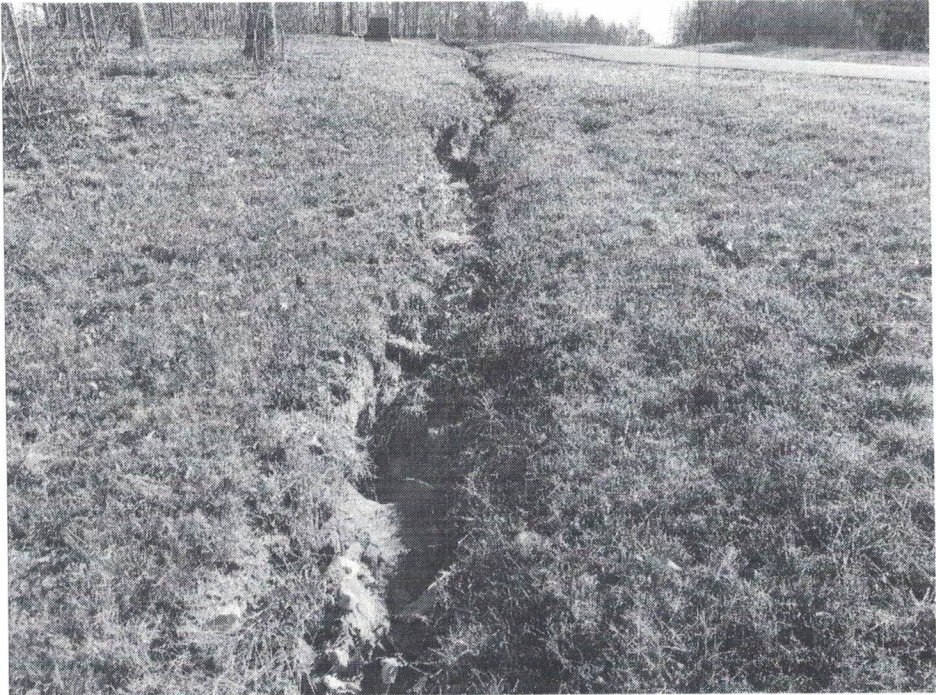
Photo 5: Outfall S208 A roadside swale was observed. The swale appears to be downcutting, and should be stabilized. Photo Taken 11/30/2023
