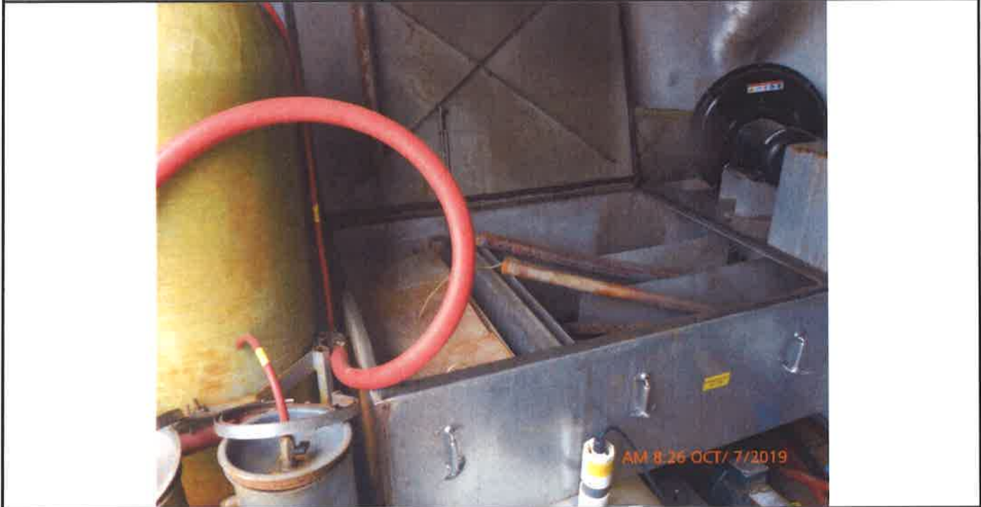
Photo 1. View of the North Deactivated Dual Phase Extraction System (DPE).
