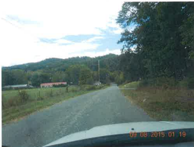
Gray spot discoloration on Stanfield Road
