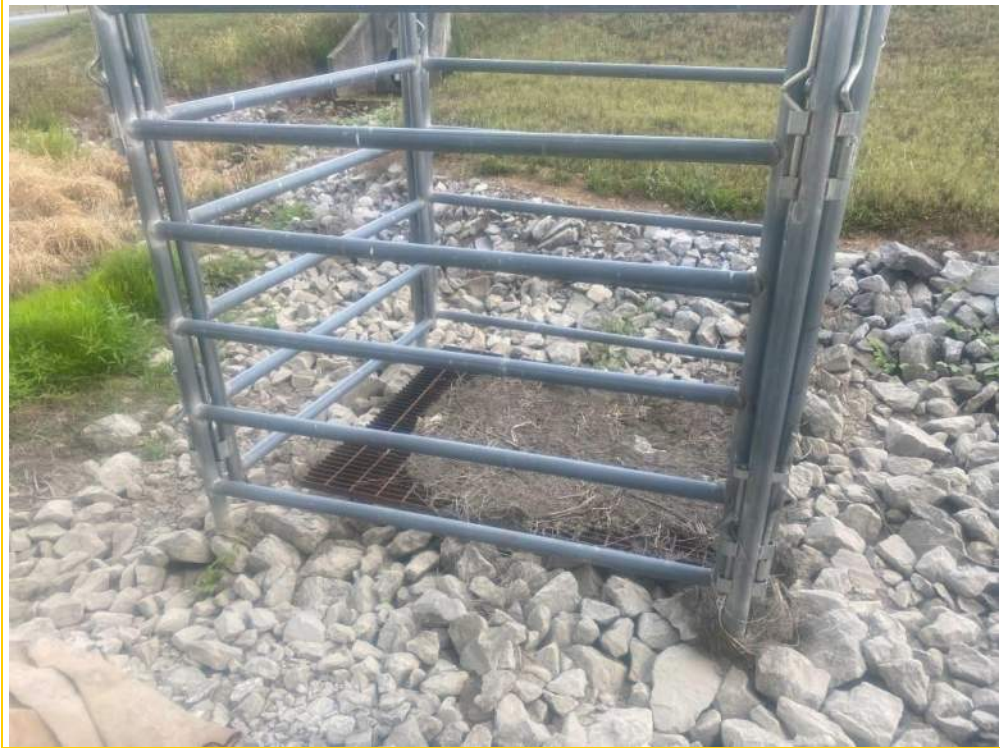
Photo 5 – General view of the inlet junction box which houses the inlet of the 48” CMP proposed for replacement.
