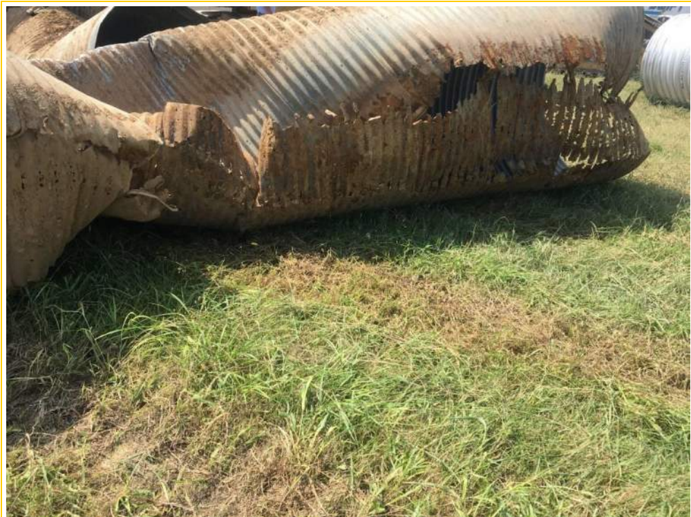
Photo 6 – Deteriorated condition of 60” CMPs after removal, permitted under NR 1903.124, located downgradient of impact proposed in this application.
