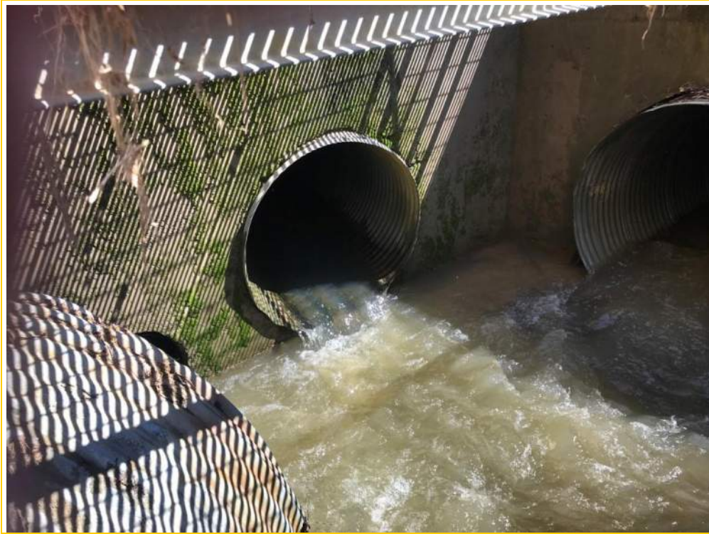
Photo 1 – Outlet of the 48” CMP proposed for replacement. The 48” CMP outlets to a junction box where it connects to 2 @ 60” CMPs.
