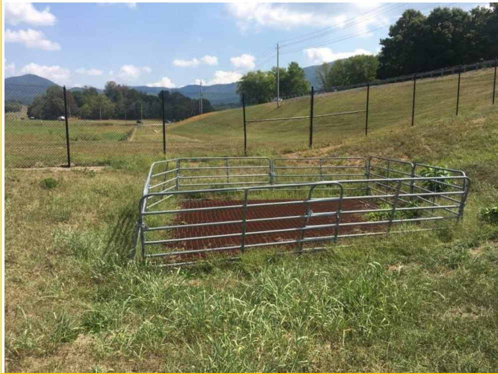
Photo 3 – Aboveground view of the junction box where the 48” CMP outlets and discharges to 2 @ 60” CMPs.
