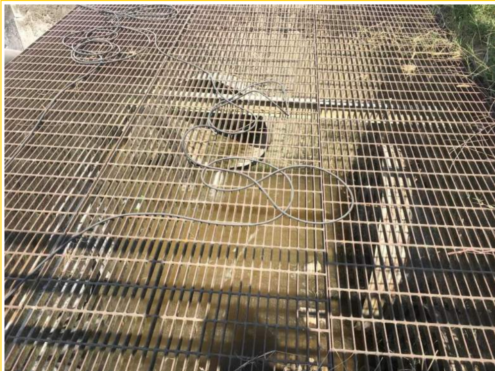
Photo 2 – Outlet of the 48” CMP proposed for replacement. The 48” CMP outlets to a junction box where it connects to 2 @ 60” CMPs.
