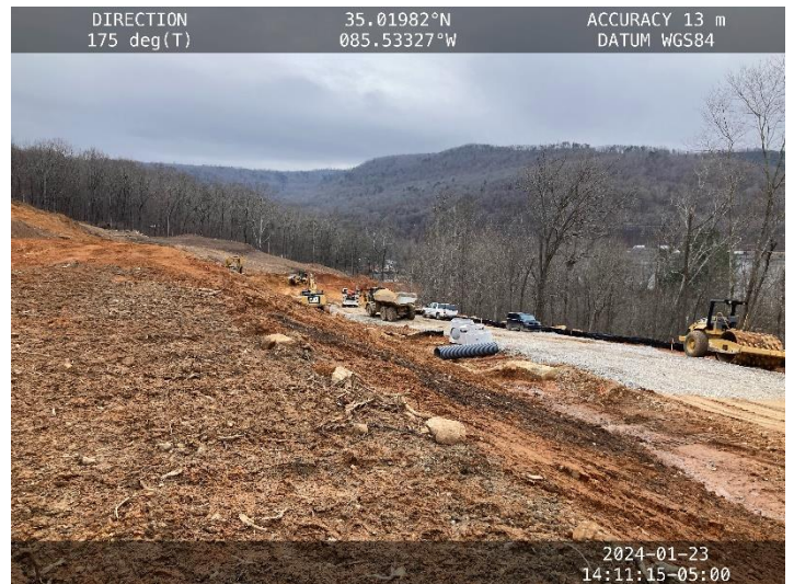
Photo 12: Facing down slope on east side of road where check dams are proposed on plans.
