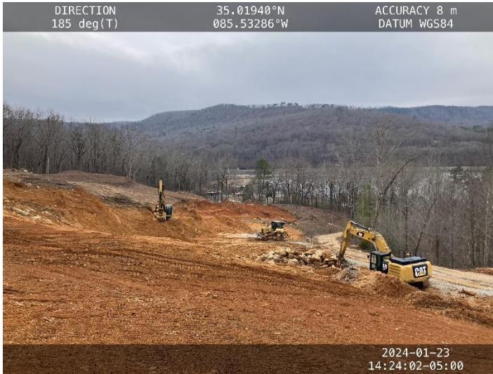
Photo 9: Facing down access road (below basin) towards recently excavated depression to temporarily help with sediment control.
