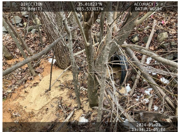
Photo 4: Evidence of sediment transport from culvert under site entrance in Photo 2 – connects directly to wet weather conveyance in sediment accumulation in Photo 3.
