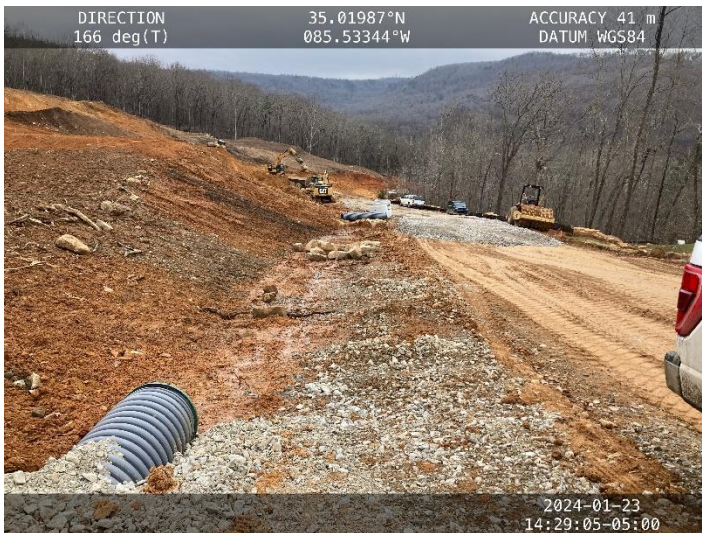
Photo 7: Facing south along access Rd at where check dams are shown on EPSC sheets.
