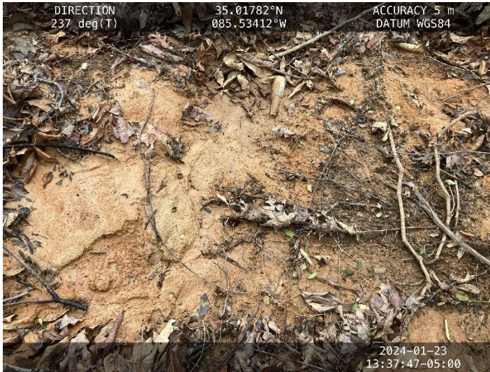
Photo 5: Evidence of off site sediment accumulation in WWC.
