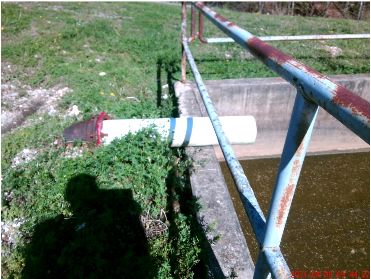
Image 2 - Plant Bypass/Overflow Pipe
