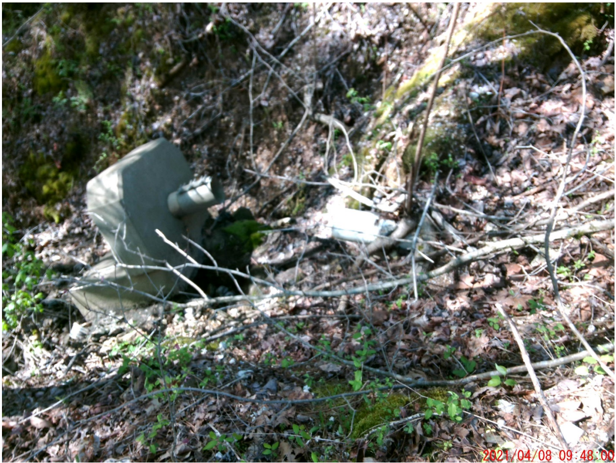
Image 4 - Discharge Pipe severed at collar (no adverse impact)
