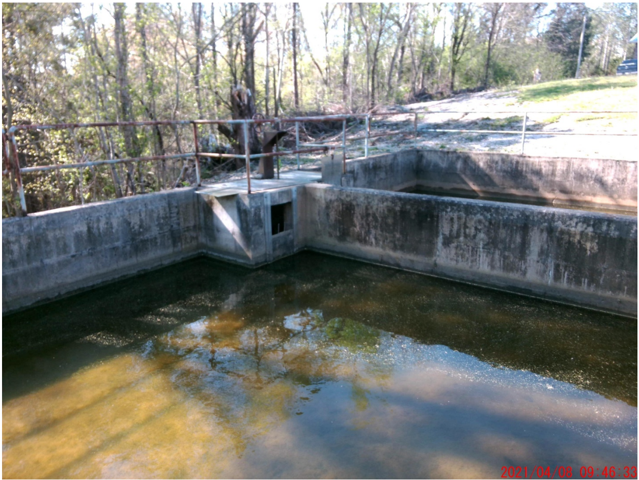
Image 3 - Discharge Gate in Lower Basin
