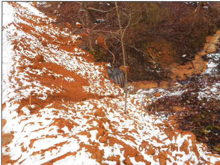
Photo 2: Sediment from crossing has entered the tributary.
