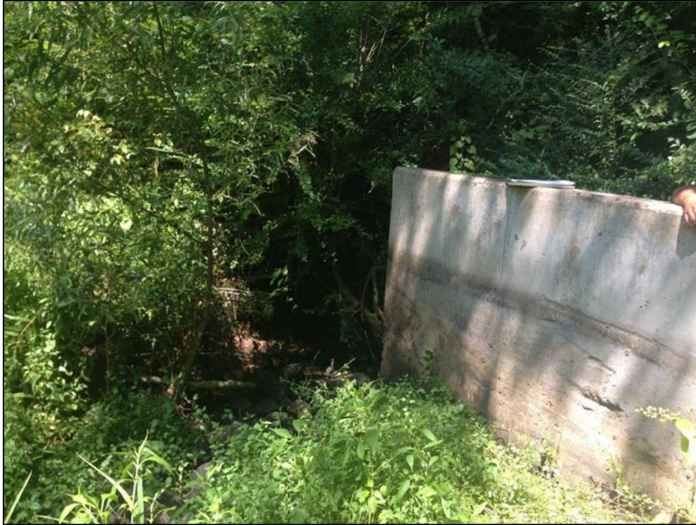
Photo 1. View looking at left side of pond dam where the stream has cut around the structure.
