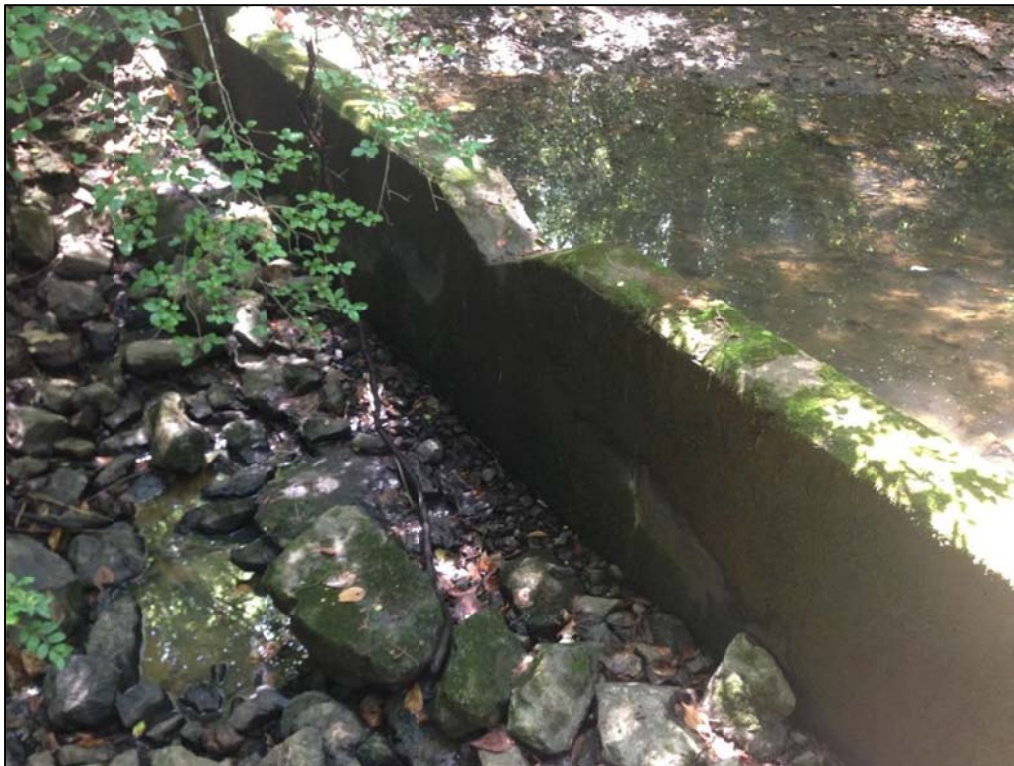
Photo 4. Another view looking upstream at the second structure and the v-notch weir. Notice the standing water upstream of the structure and that the flow is not going through the weir opening. Instead it is flowing through the rock on the left bank, which is depicted in Photo 3.
