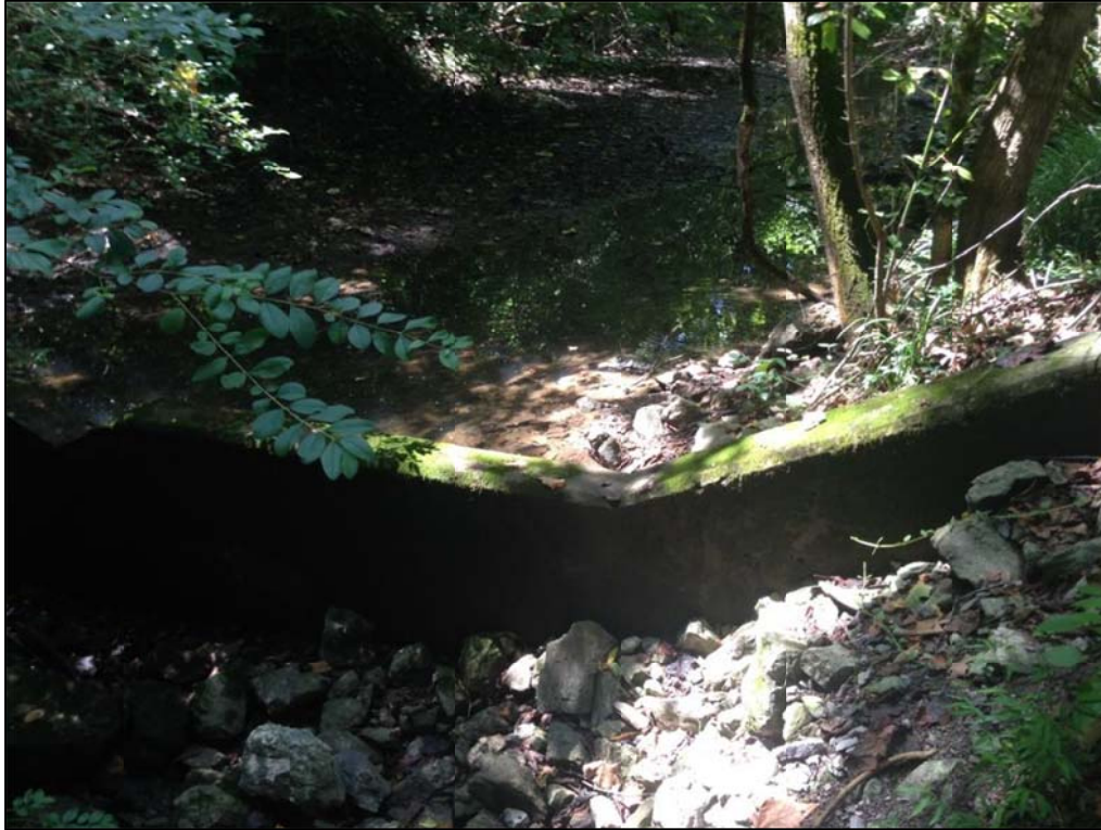
Photo 3. View looking at second (downstream) weir/dam structure where it interfaces with the left bank.
