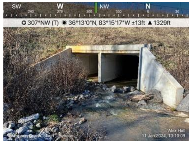
Photo 4: PS 14 (Thompson Creek) culvert facing northwest looking downstream. Not associated with this project.
