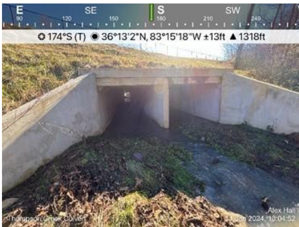
Photo 3: PS 14 (Thompson Creek) culvert facing south looking upstream. Not associated with this project.
