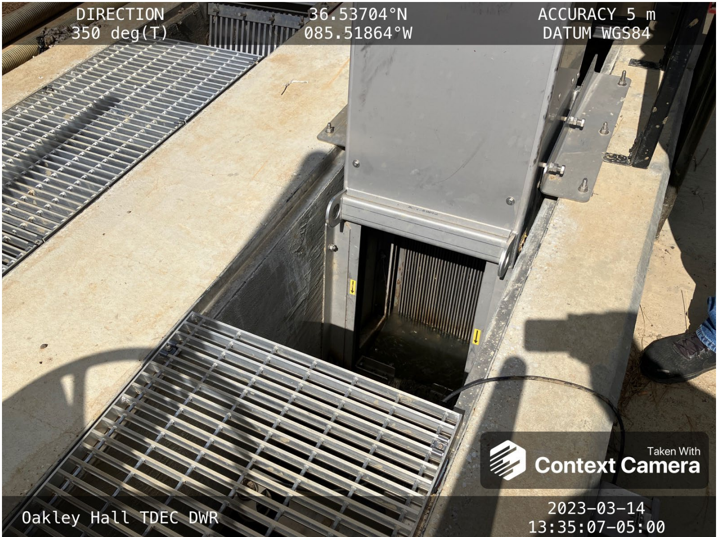
The screens were operable. This was an important improvement to the system.
