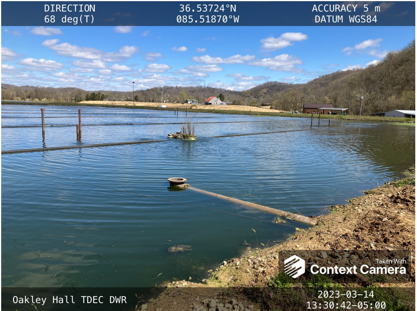
The discharge from the headworks to the first lagoon is pictured. It is entering the lagoon through the bottom of the pipe.
