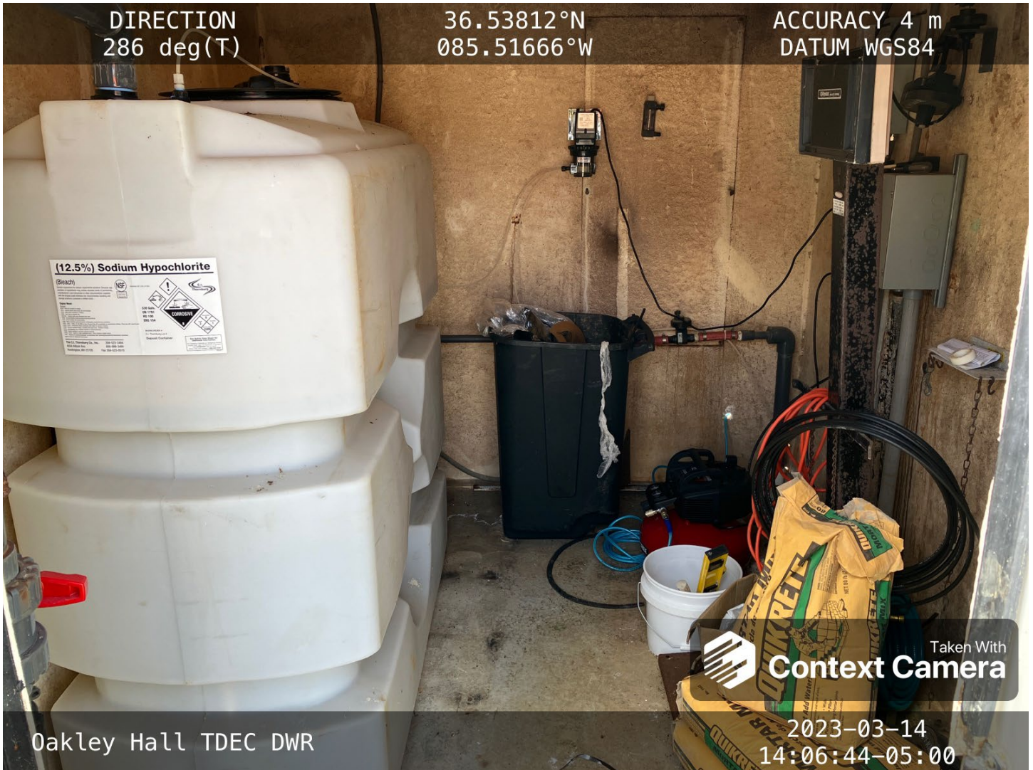
The bleach tanks and dosing pump were reviewed and found to be in operation.
