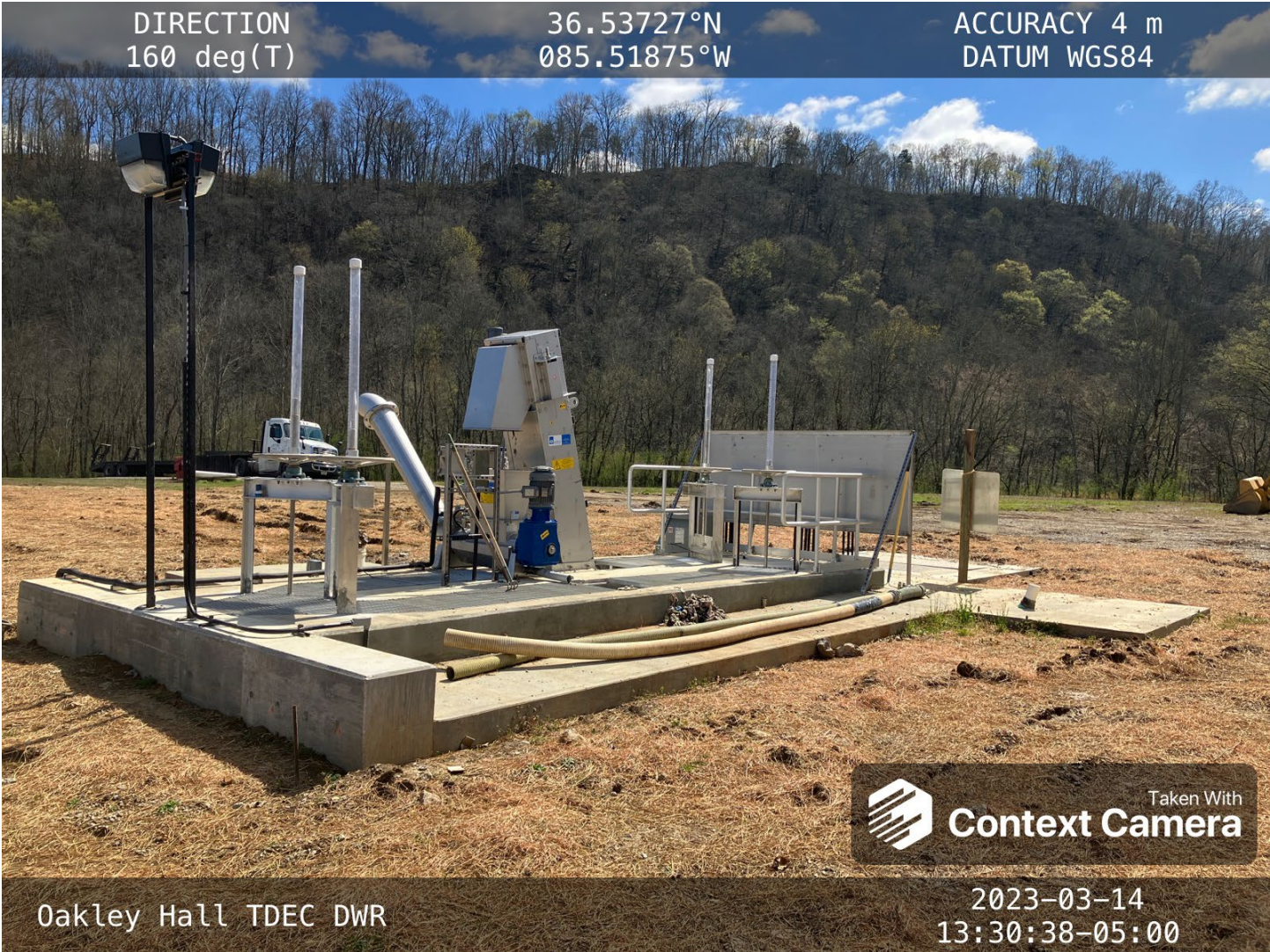
The new headworks is in place. Some landscaping work is still in process.
