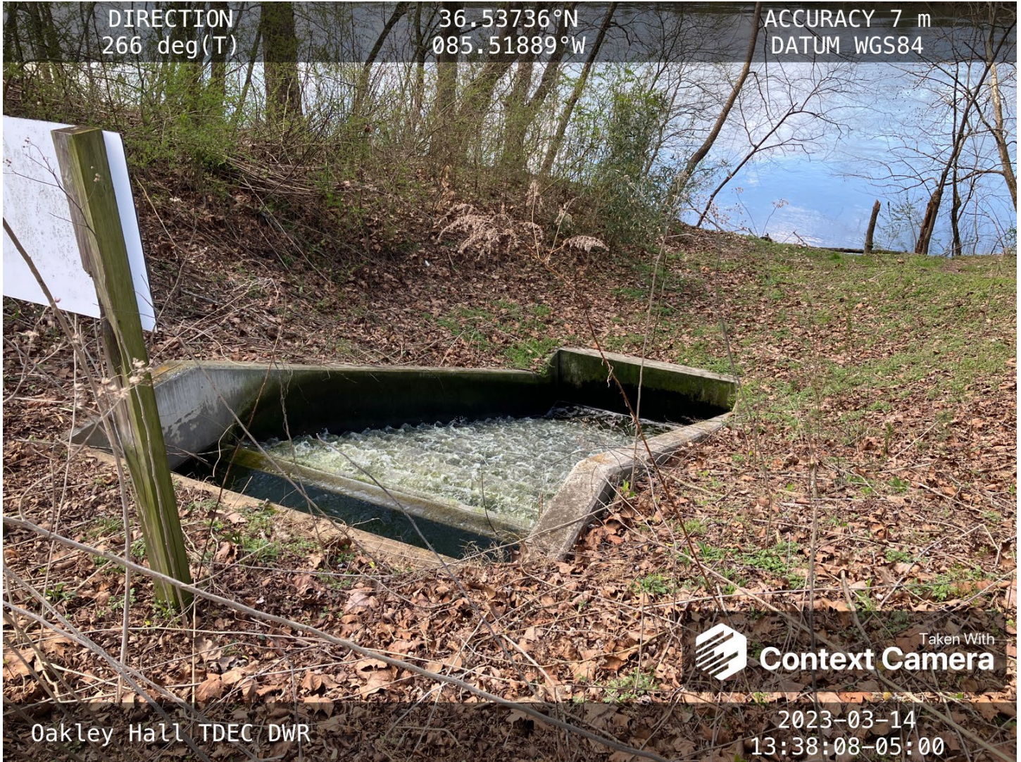
The effluent outfall to the Cumberland River is pictured.
