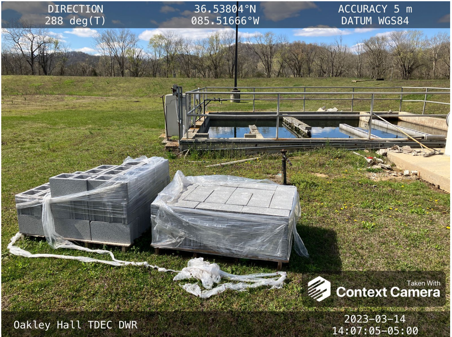
Block work is being prepared for the Chlorine Contact Chamber. Some block has been laid, most with no mortar This was explained by the operator so to see how the process is going to work out.
