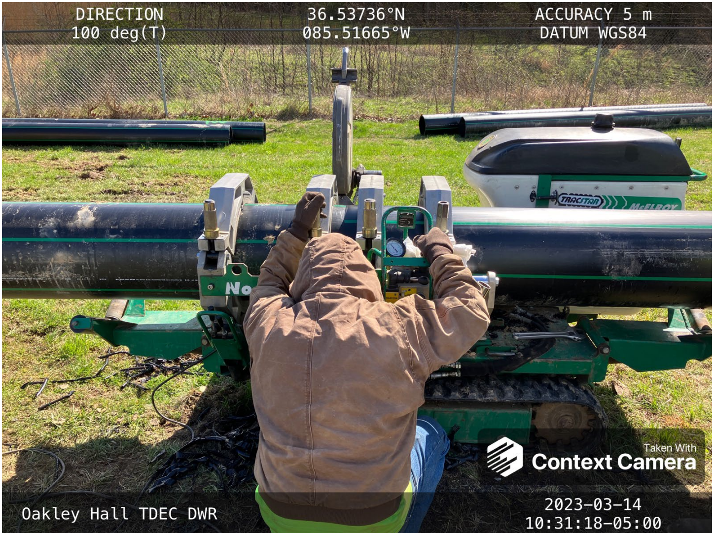
One of the flush heated pipe connections of the poly pipe was observed. The connection process and strength were discussed with the contractor.
