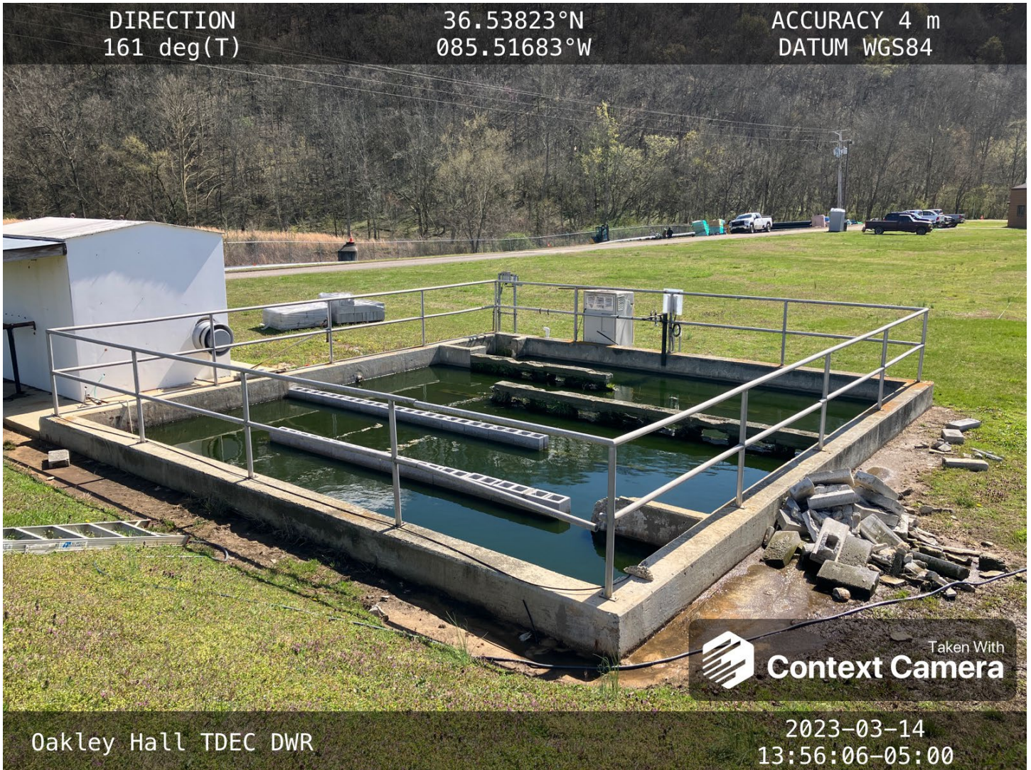
Operators have started the block work on the chlorine contact chamber. Mortar has only been tested on a few of the block.
