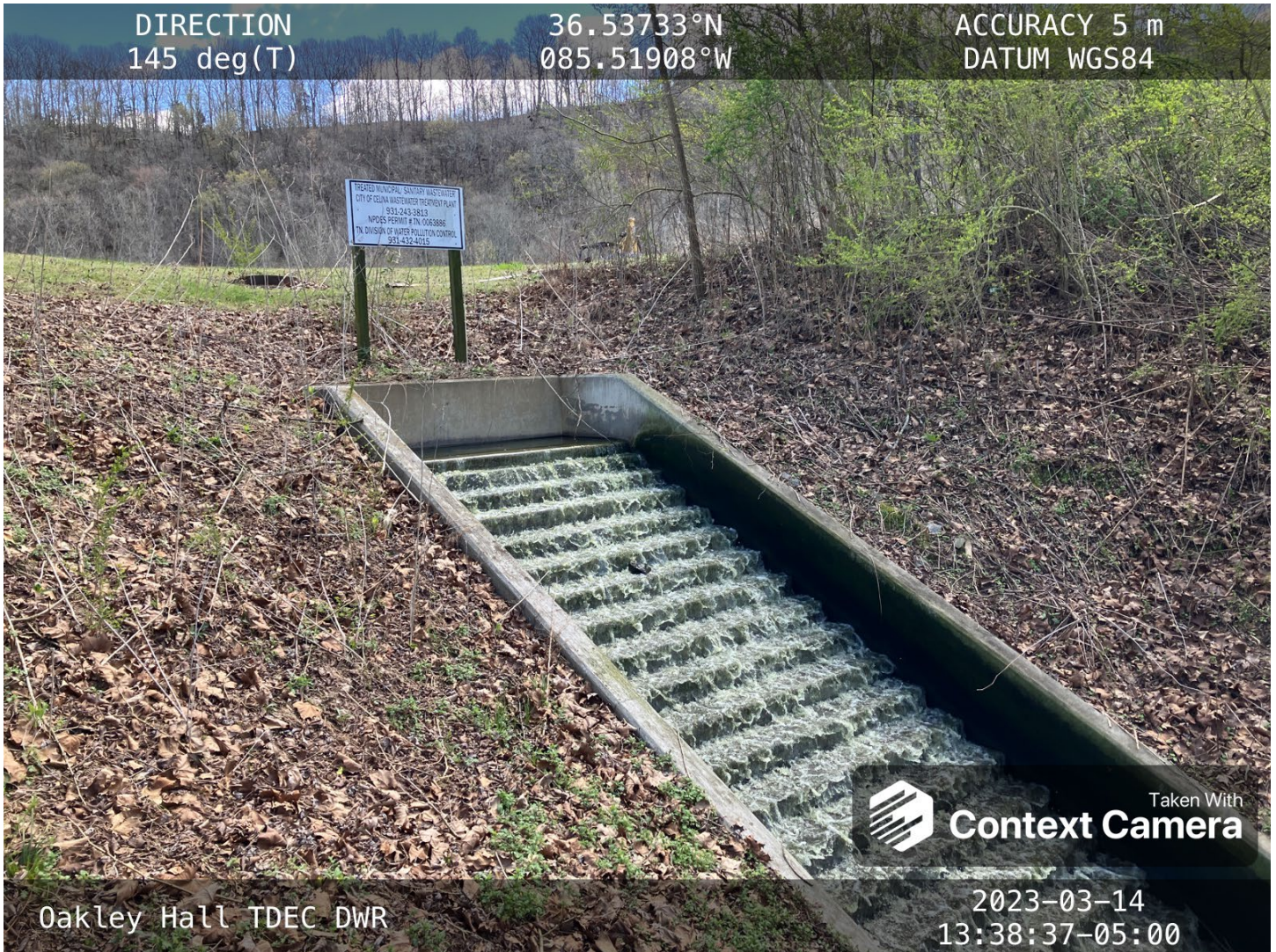
The effluent aeration steps are pictured (just above the outfall). A slight green color from algae was observed.
