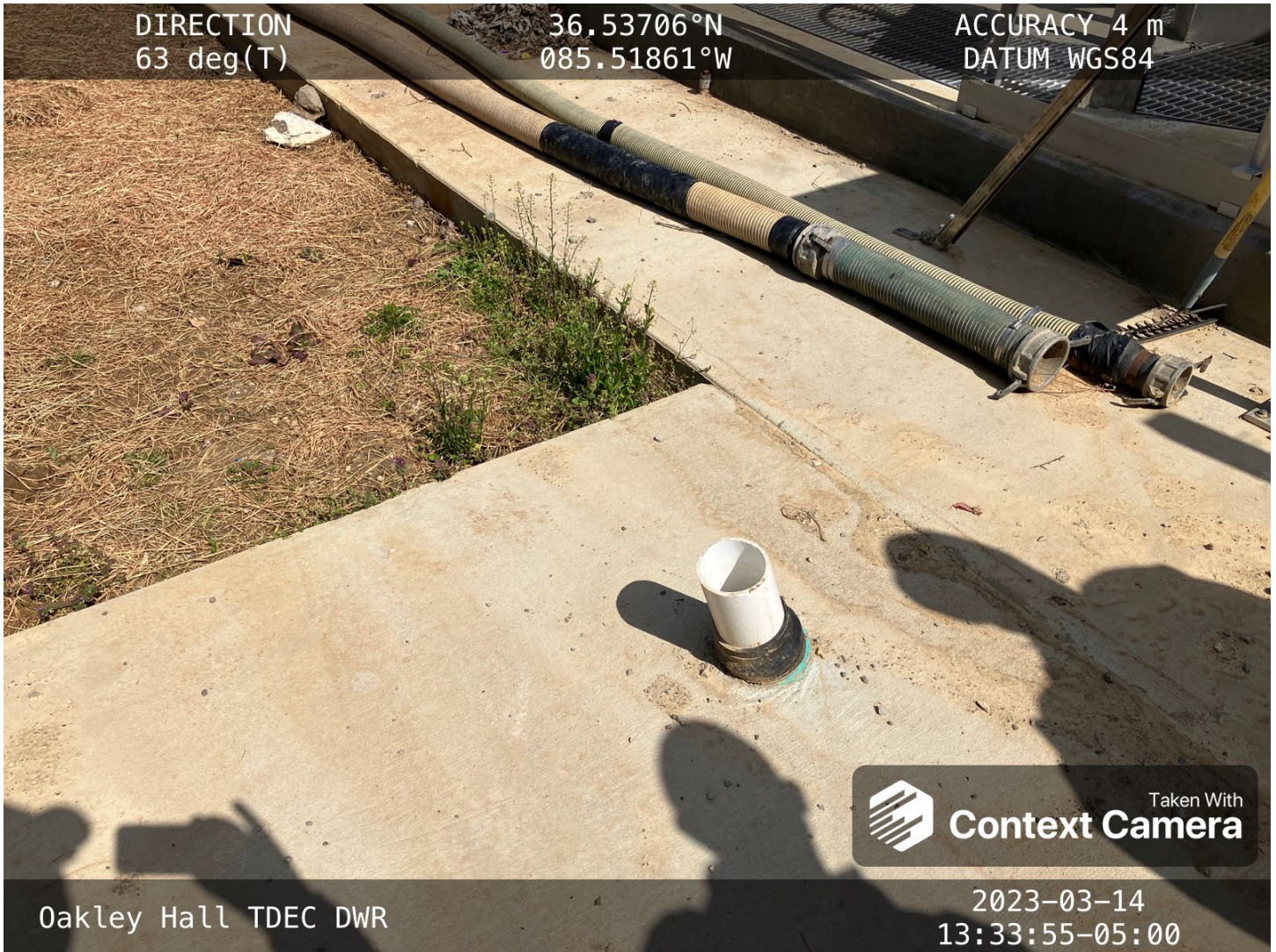
A pipe is configured to add wastewater into the system. This port is after flow measurement and cannot be used to except septage waste brought in from offsite, e.g., marina or septic tank waste. This port should be capped.
