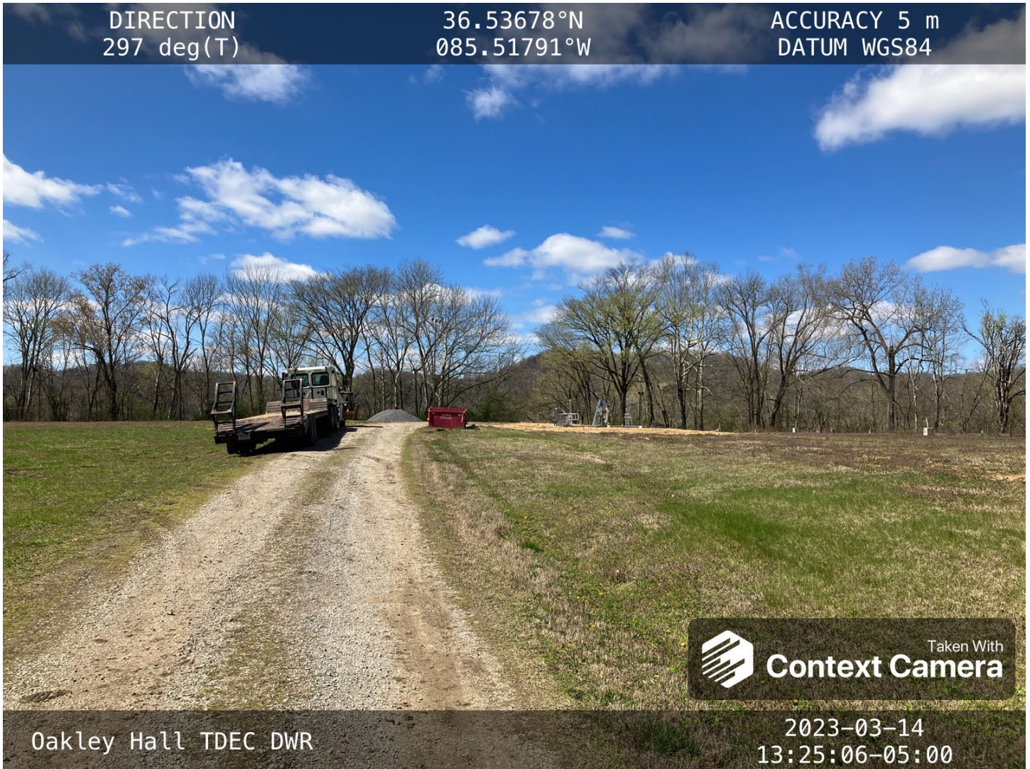
Construction of the mechanical and electrical equipment is mostly complete. The entrance road is in good condition.
