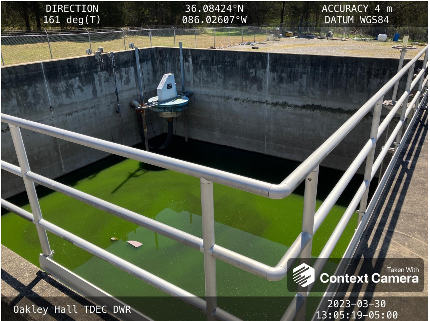
The inoperable reactor is dormant. Seals and other equipment may need further work.
