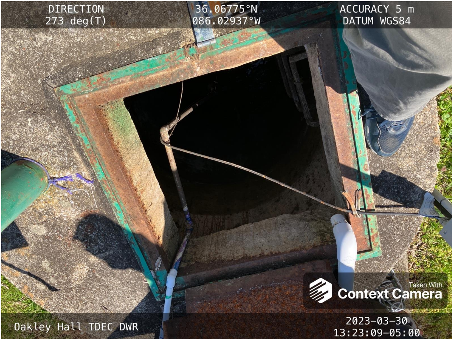
The pump station wet well was observed. The well was clean with a minimal amount of grease.
