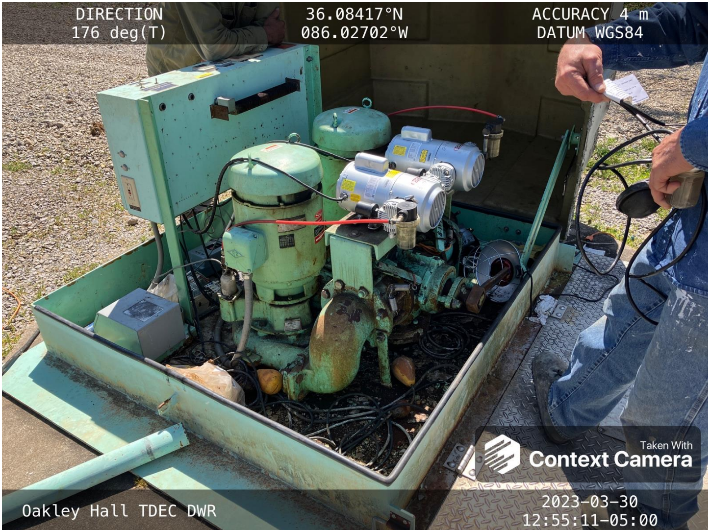
The in-plant pump station was in operation.
