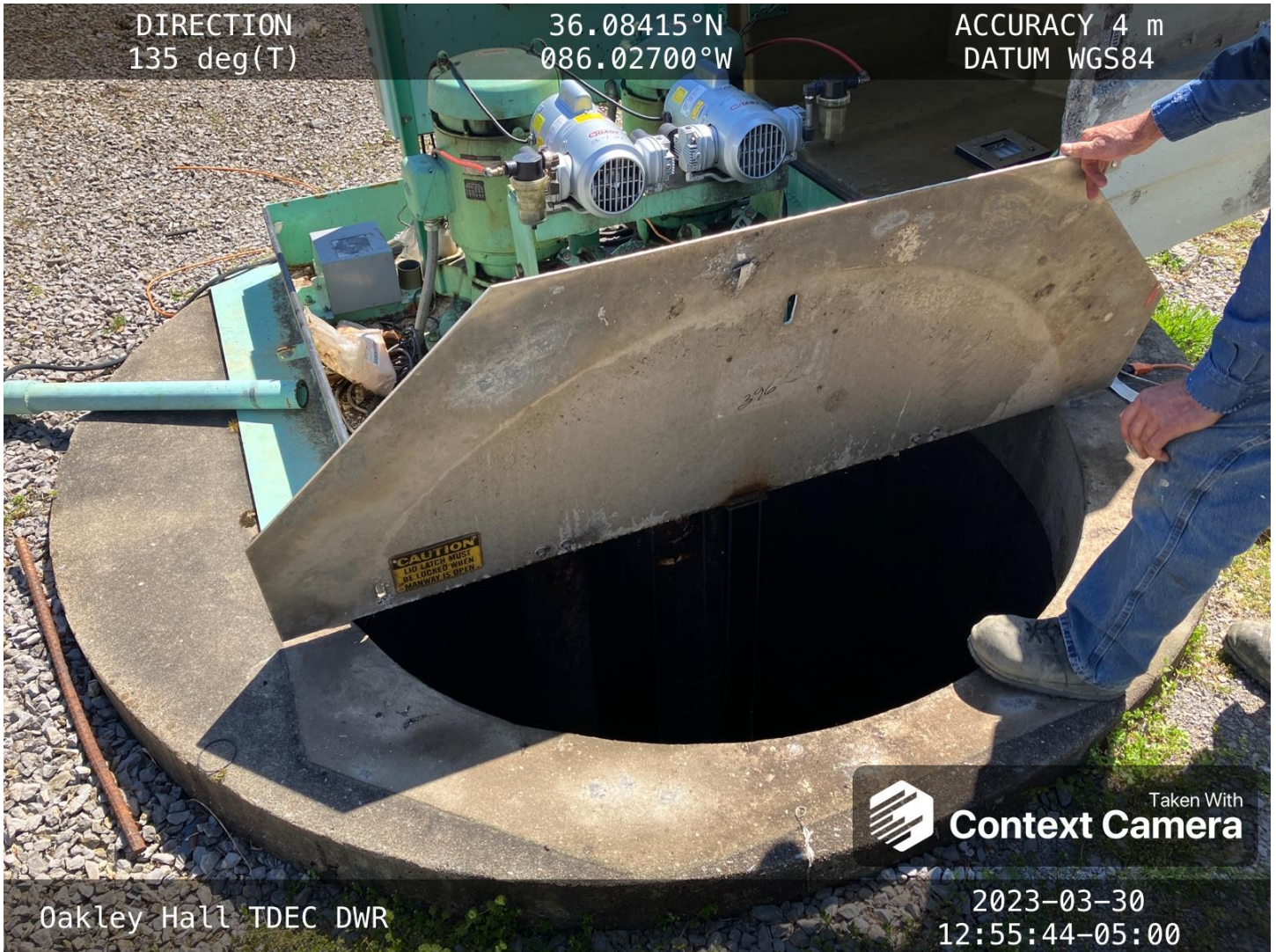
The wet well for the pumpstation was reviewed. Grease was not present in the wet well.
