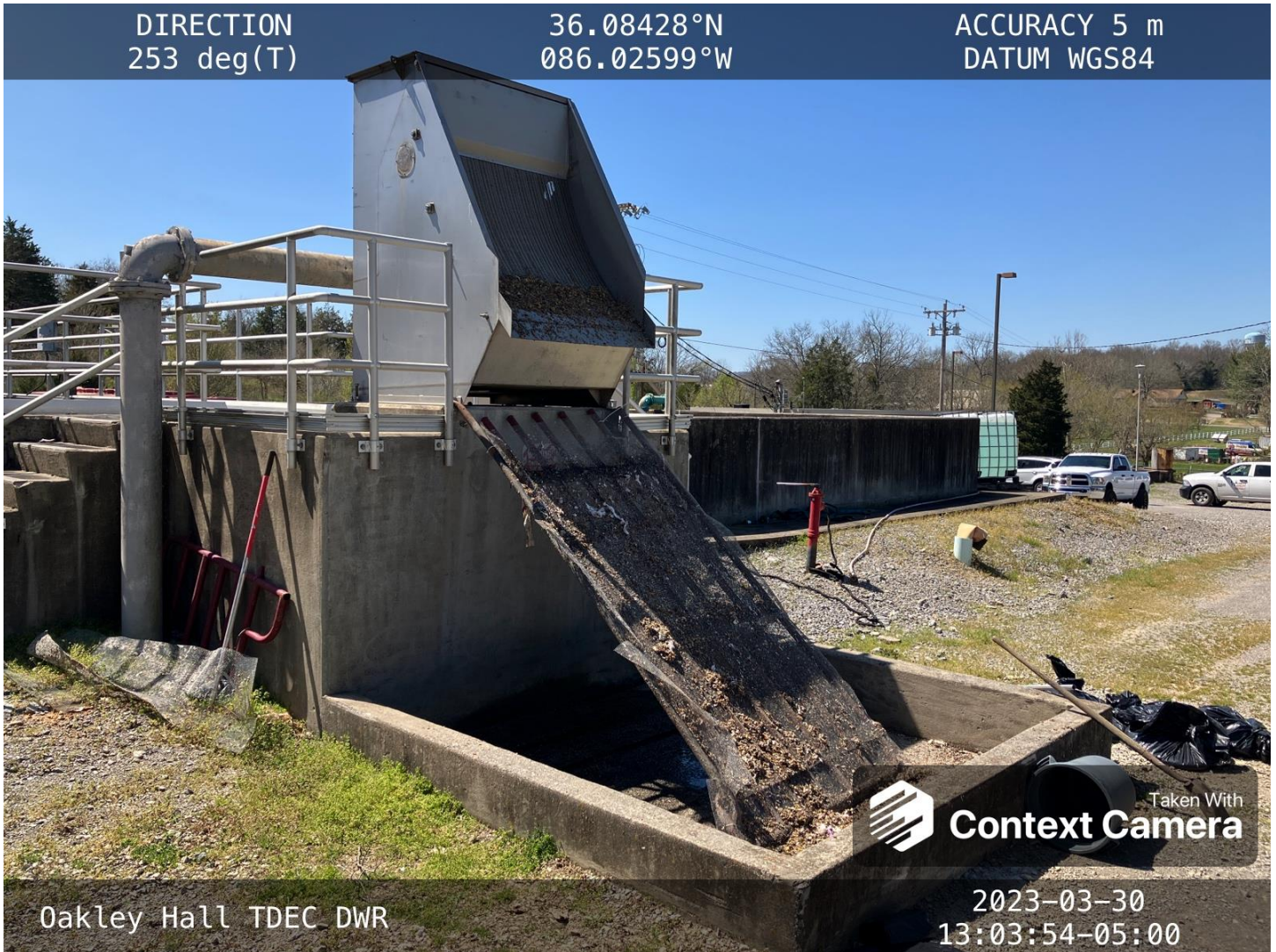
The influent screen is operational. Solids are raked and bagged. They are disposed of in the landfill.
