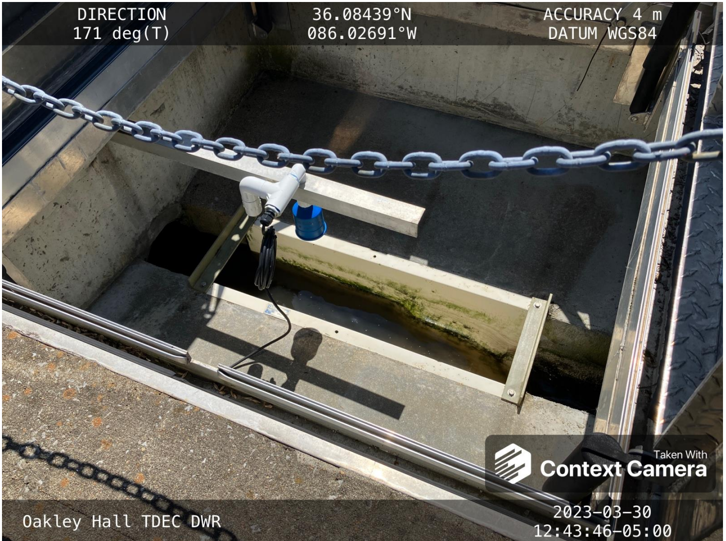
This effluent flume (Palmer-Bowlus) is pictured. The effluent discharge flowing through the flume was dark due to the suspended solids in the discharge.
