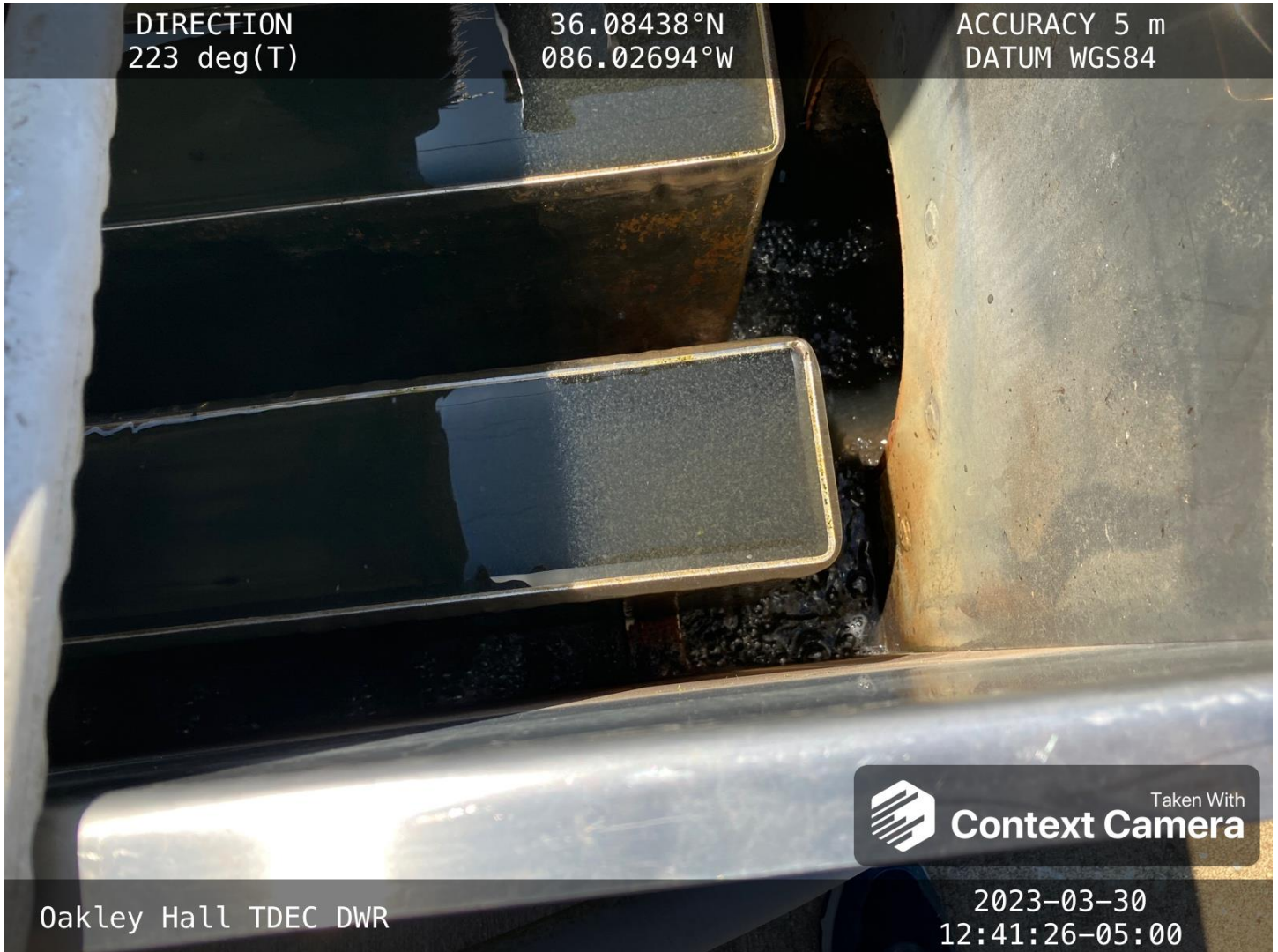
At the Ultra Violet (U.V.) system discharge, it was observed that suspended solids were present.
