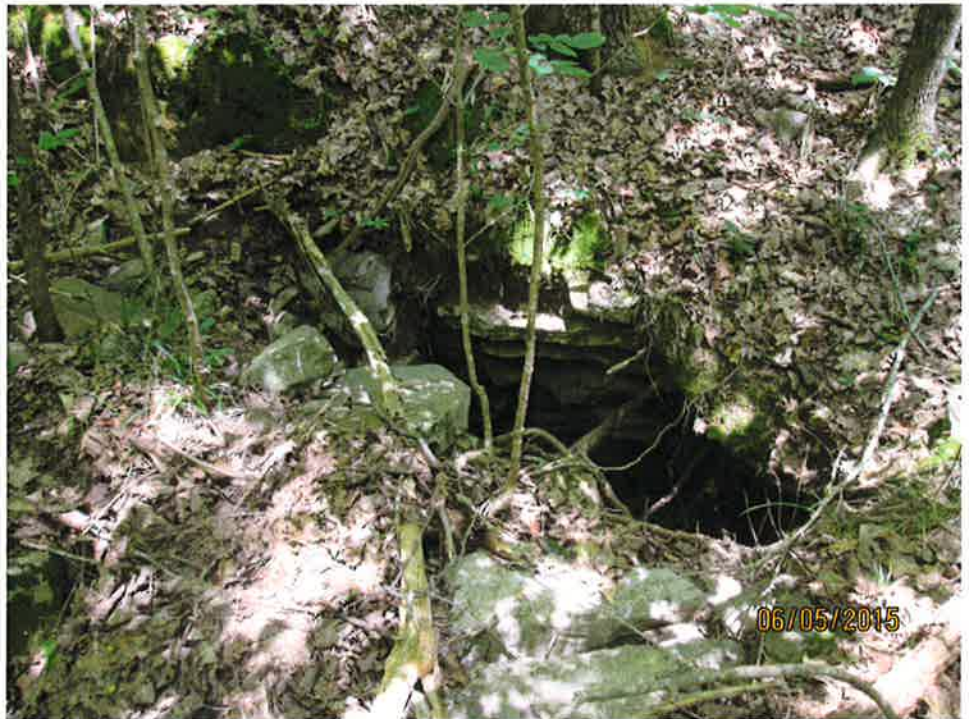
Photo 4: Opening of Cave in Channel B Upstream of Evaluated Segment Photo Taken 6/5/2015
