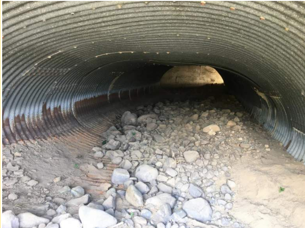
Photo 3 – General view of interior of the single 60” CMP. CMP is noticeable misshaped and disjunct. This pipe conveys Clear Creek.
