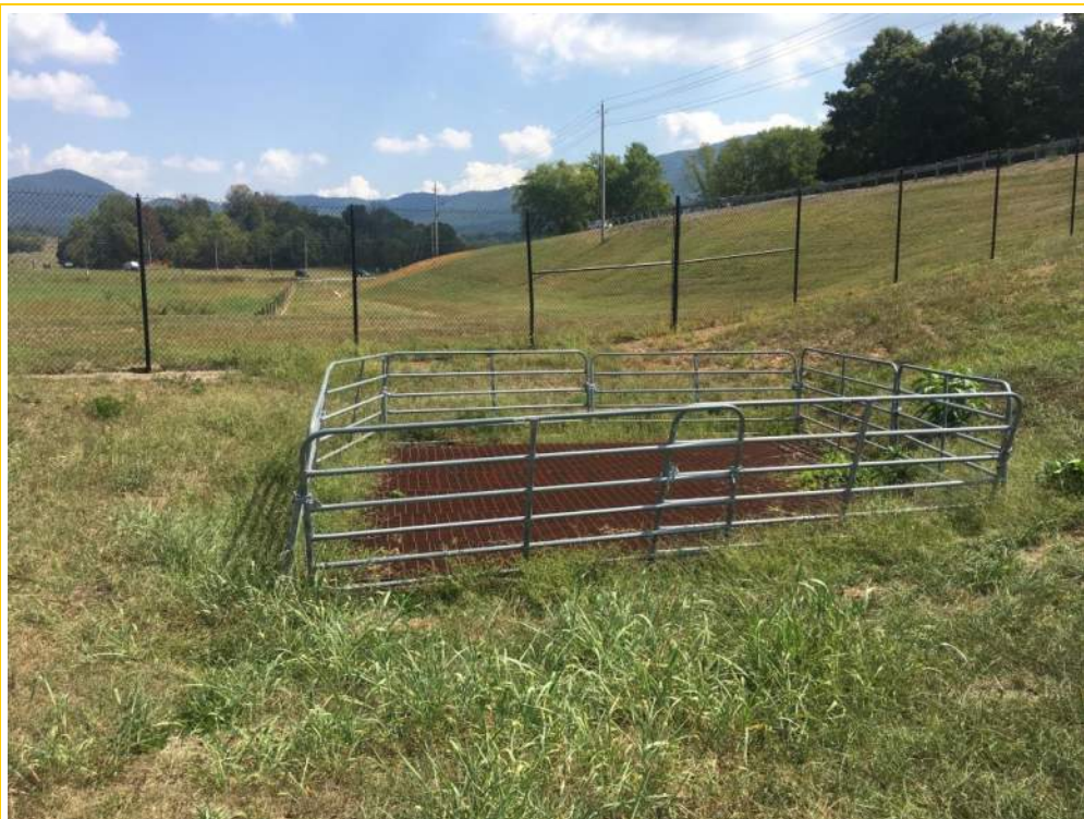
Photo 4 – General view facing upgradient of upstream junction box; transition location from single 60” CMP to two 60” CMPs.
