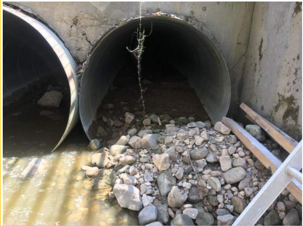
Photo 7 – General view of the outlet of the two 60” CMPs proposed for replacement as part of the modification. Debris build up was evident and culverts were observed to be damaged and disjunct.
