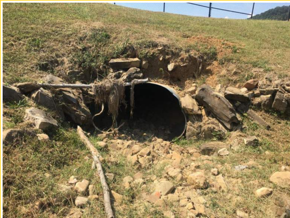
Photo 2 – General view of existing one 60” CMP at inlet. CMP is partially collapsed; surrounding area shows sign of erosion; debris build-up evident. Proposed begin impact location for permit modification request.
