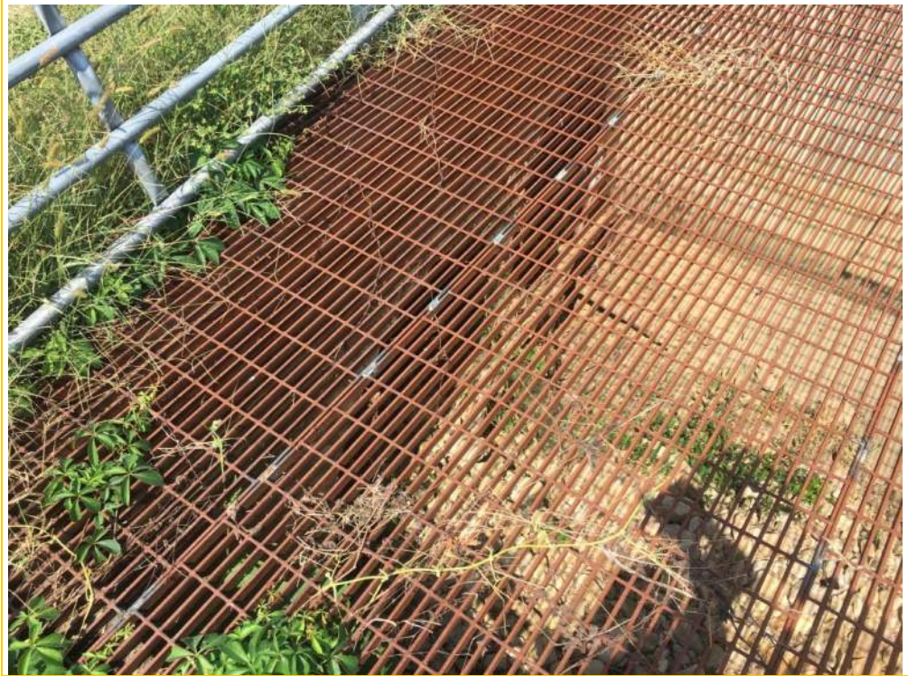
Photo 5 – General view of the inlet of the two 60” CMPs at the upstream junction box.
