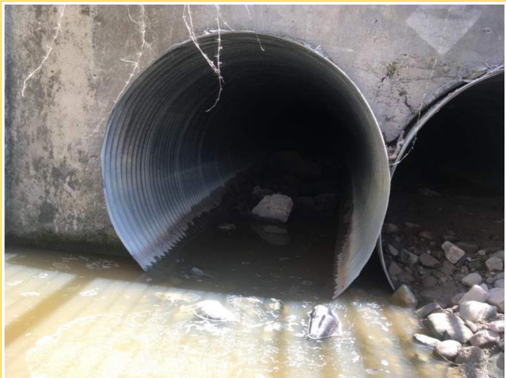
Photo 8 – General view of the outlet of the two 60” CMPs proposed for replacement as part of the modification. Debris build up was evident and culverts were observed to be damaged and disjunct.
