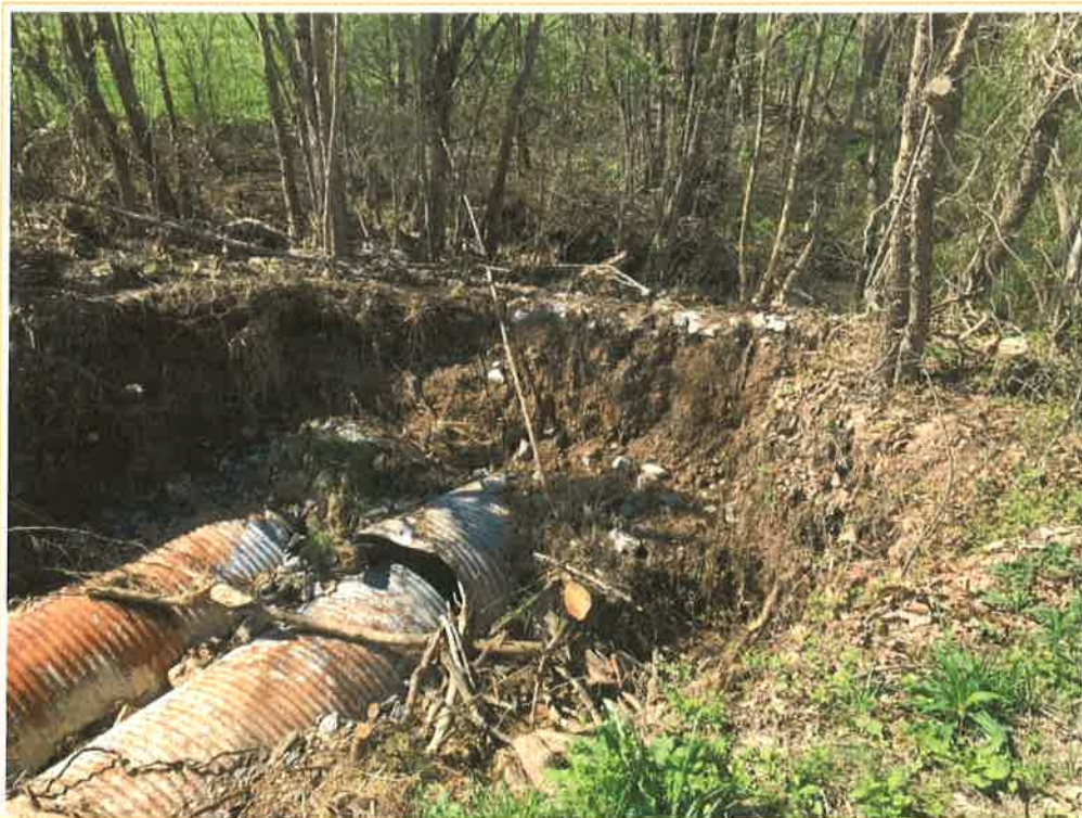
Photo 4 – General view of damaged 60” CMPs facing downstream, immediately upstream of the outlet headwall.
