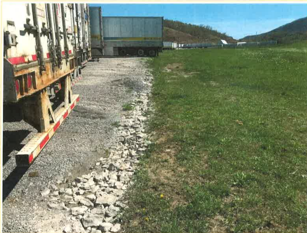
Photo 9 – Gravel parking lot and riprap side ditch/French drain upgradient of the collapsed area.
