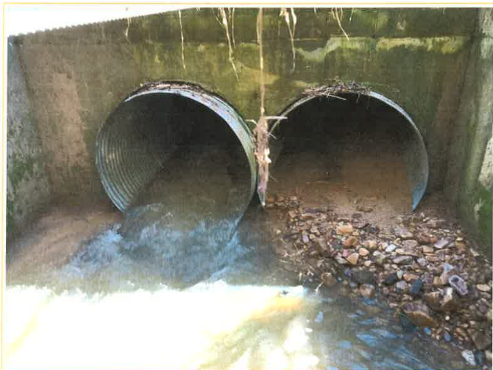
Photo 12 – View inside the junction box, showing two of three CMPs that enter this junction box. These two CMPs convey Clear Creek.
