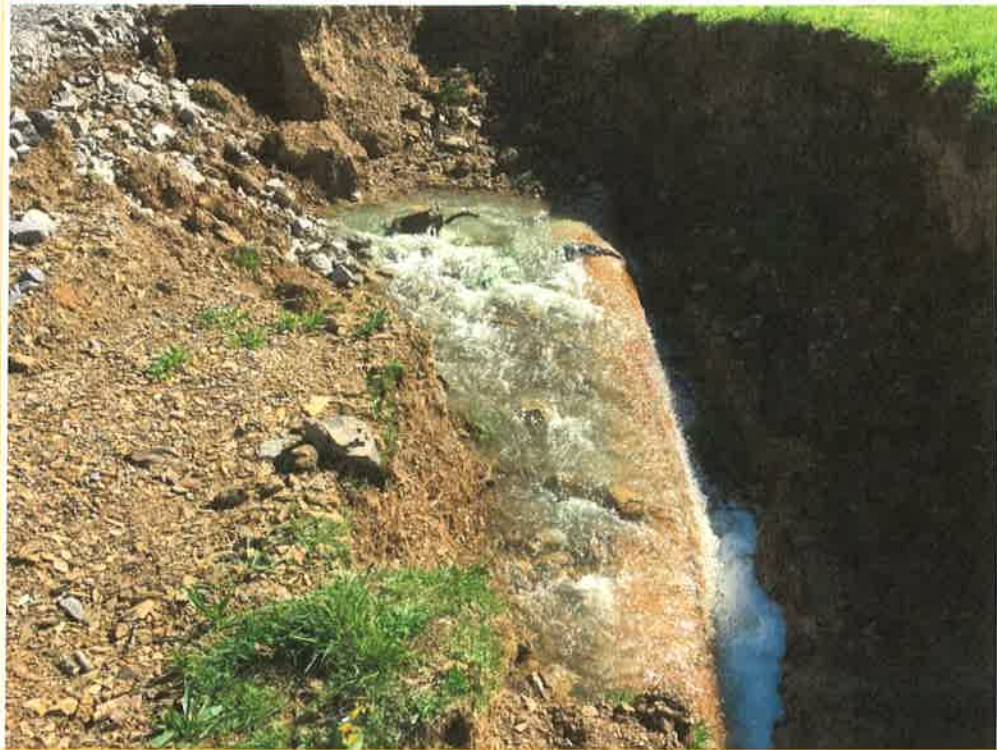
Photo 7 – Beginning of the collapsed pipe area, stream was observed escaping from the culverts. Normal flow conditions.
