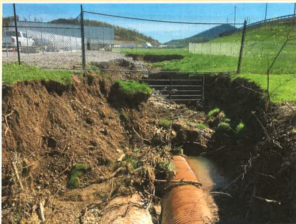
Photo 2 – Looking upstream from headwall at collapsed area. CMPs are disconnected, deteriorating and permanently damaged. Collapsed area is approximately 6 to 8 feet deep.
