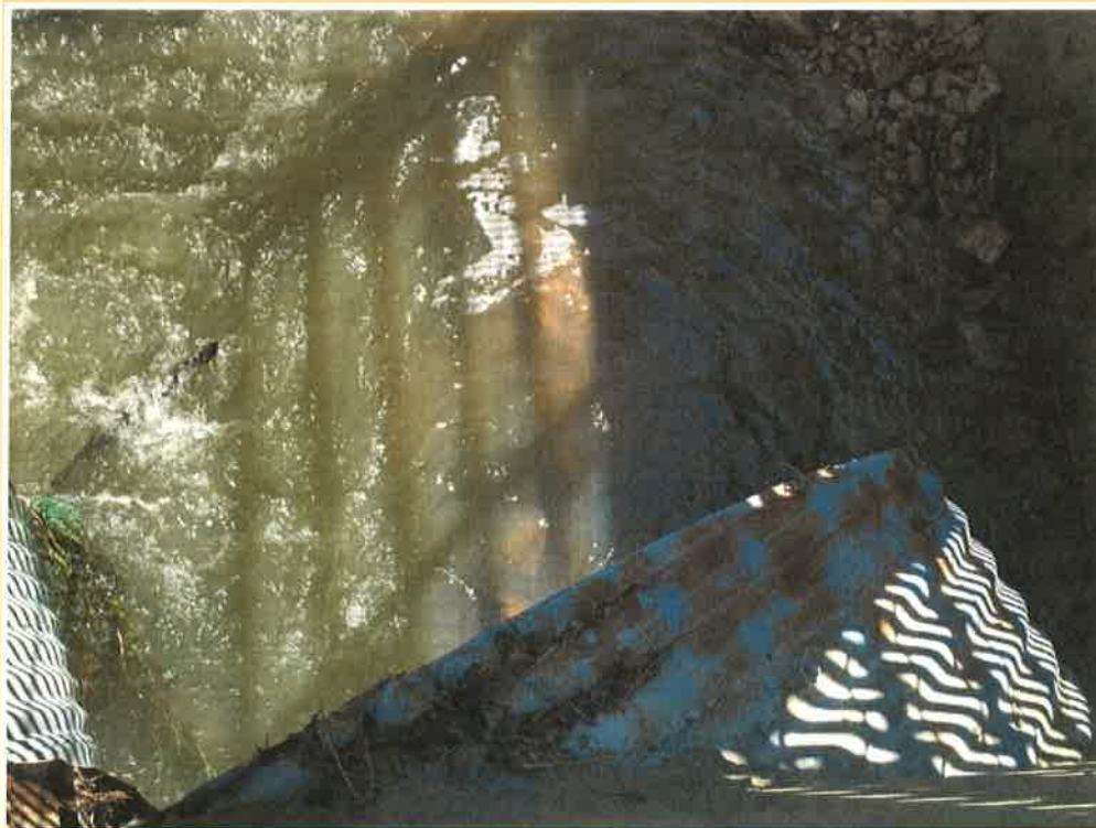
Photo 14 – View of the outlet CMPs inside the junction box. These pipes are proposed for replacement, if needed.
