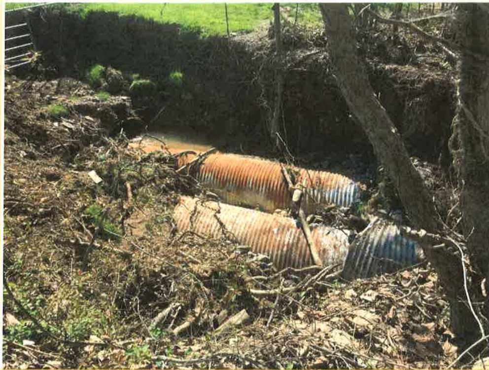
Photo 3 – General view of damaged 60” CMPs immediately upstream of the outlet headwall.
