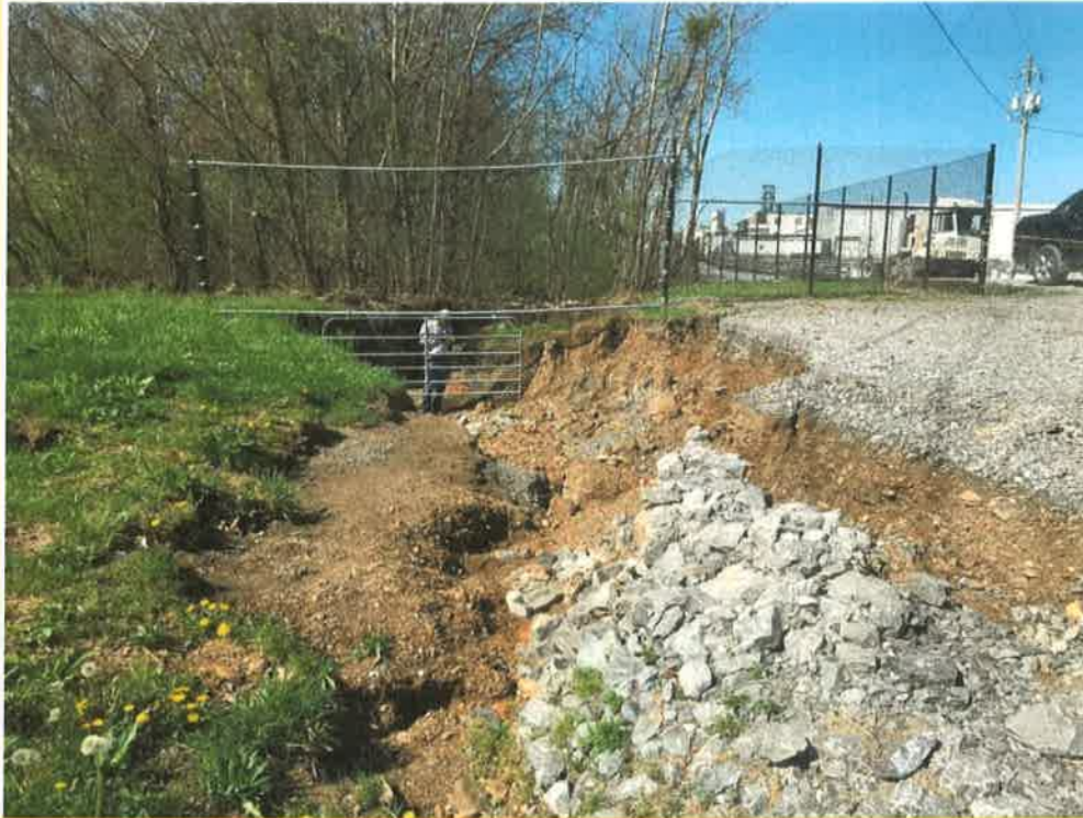
Photo 5 – General view of collapsed area, approximately 100 ft upstream of the outlet headwall. A portion of the gravel parking lot and riprap side ditch/French drain is damaged and evident in this photo.
