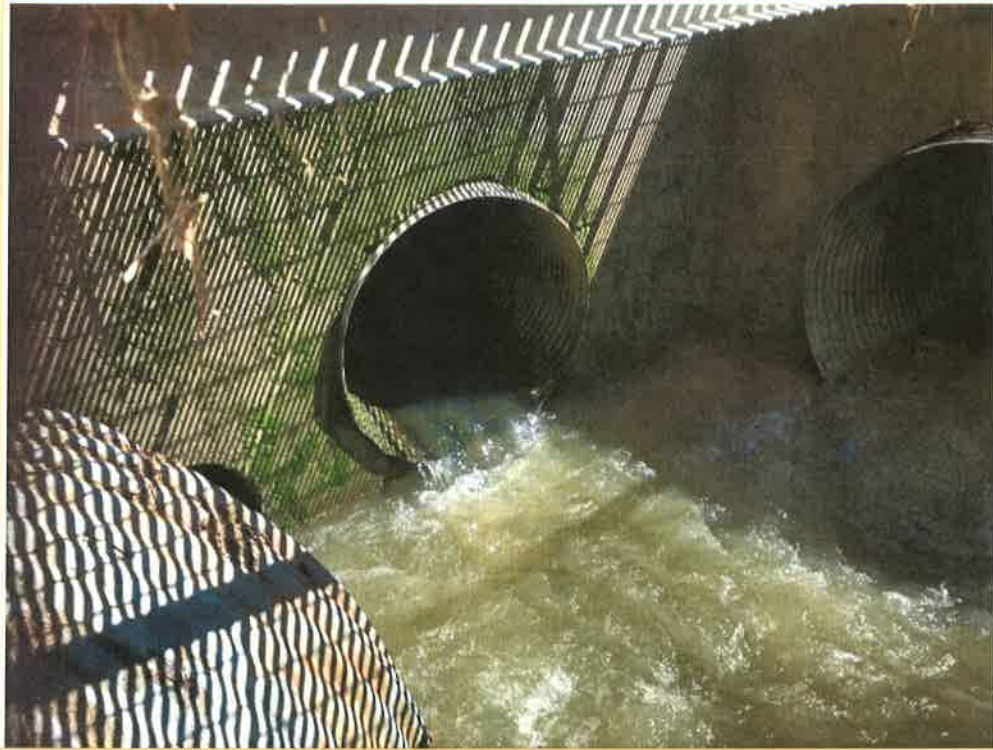
Photo 13 – View of the third CMP entering the junction box. This junction box will be used to begin the stream diversion/pump around since it is a stable, accessible location.
