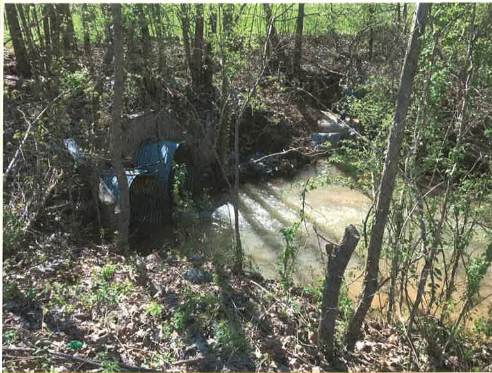
Photo 1 – Outlet of 2 x 60” CMPs and concrete headwall. The headwall is in good condition and is not proposed for preplacement. End of proposed impact location.
