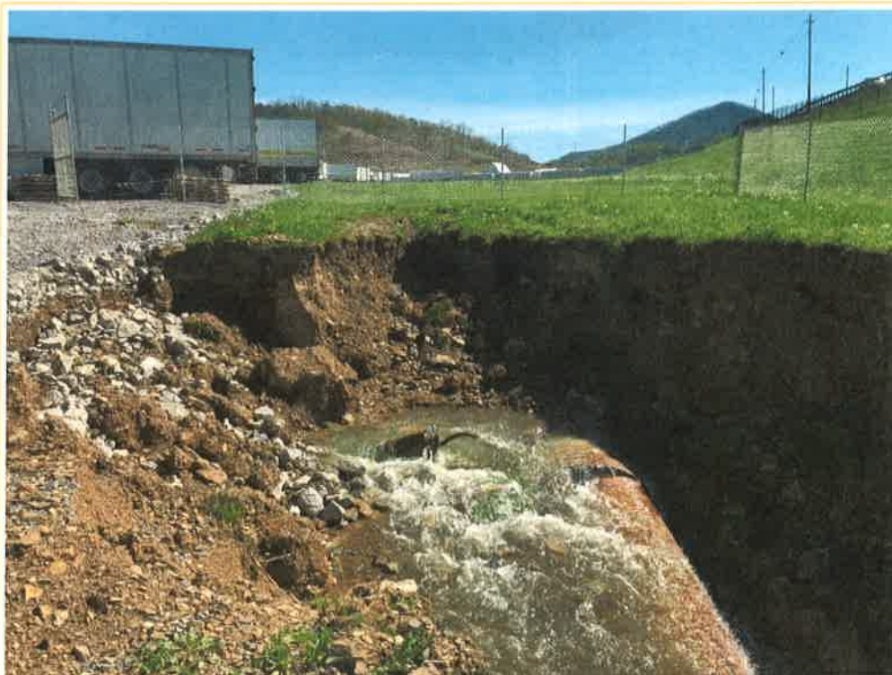
Photo 6 – Beginning of the collapsed area, approximately 156 ft upstream of the outlet headwall. The stream can be observed escaping from the culverts.
