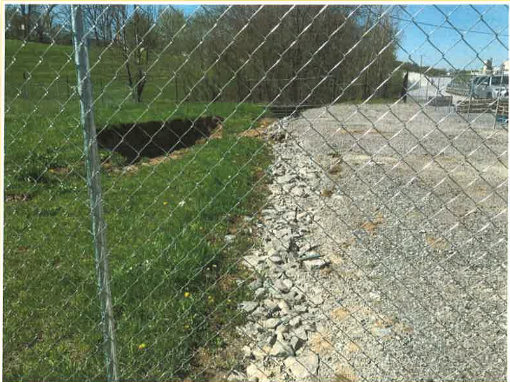
Photo 8 – General view immediately upgradient of collapsed area. Bush Brothers & Company erected a safety fence to restrict access to the area.
