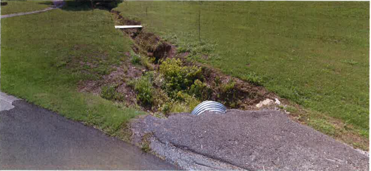
Creek Crossing 4 – Unnamed Tributary to Troy Fork Creek, Tributary to Richland Creek, Looking North East
