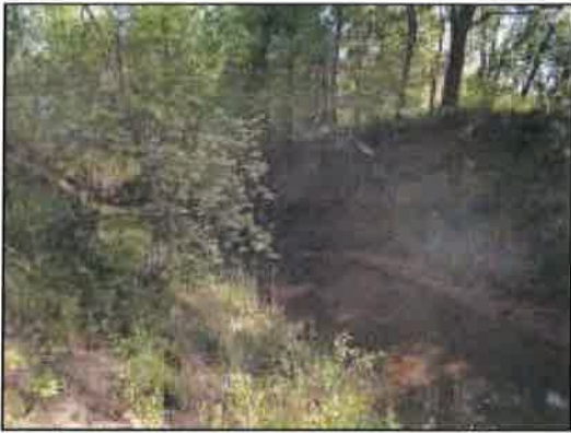
Figure 50: Looking downstream at outside bend erosion of east bank; standing on toe of the silt deposits on the inside of the bend
