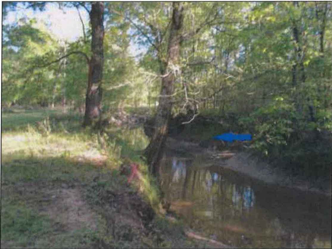
Figure 10: Just upstream of the bend looking downstream; the channel has undermined the upper bank on both sides; the blue arrow denotes the point where a wet weather conveyance discharges into the Lateral from the east
