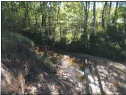
Figure 67: Slope failure of the west bank on the inside of a bend
