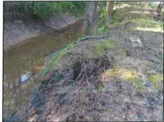
Figure 31: Close up of erosion around a root ball on the east bank
