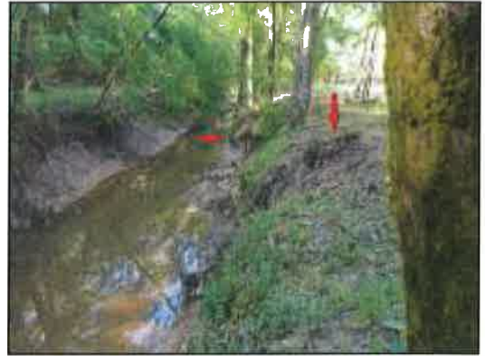
Figure 29: Looking upstream from the same vantage point as figure 28; note that east bank slope is beginning to lay back while the west bank is near vertical; the red arrows indicate where the root ball of trees have been undermined and failure is imminent
