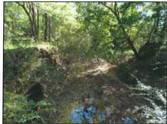
Figure 62: Looking downstream from the same vantage point as figure 61; note the near vertical slope on the west side
