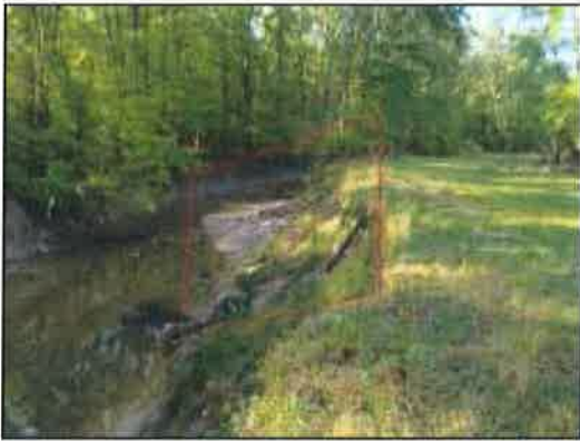
Figure 11: Looking upstream along a straight section of highly eroded bank; note the slope failure at the downstream end of the bend
