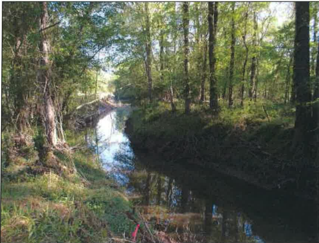
Figure 7: Upstream end of first bend looking downstream at the bank repair; note that the slope of the sloughed bank downstream of the repair is approximately the same as the slope of the repaired bank.
