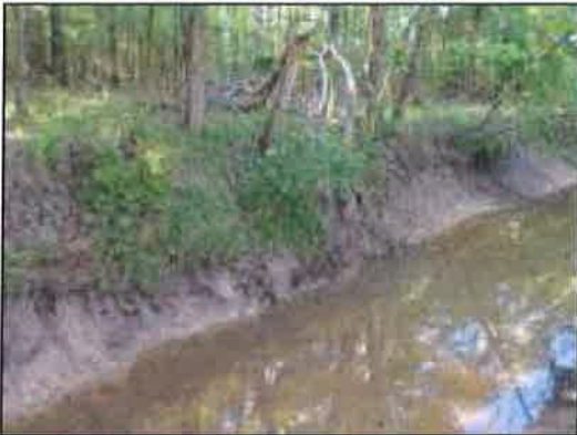
Figure 30: Undermined tree roots on the west bank
