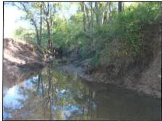
Figure 39: Standing at the toe of the slope failure of west bank looking downstream
