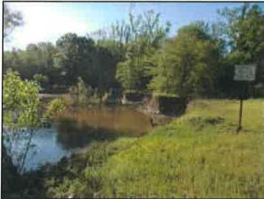
Figure 1: Standing over SS Outfall at the confluence of the Lateral with the Wolf
