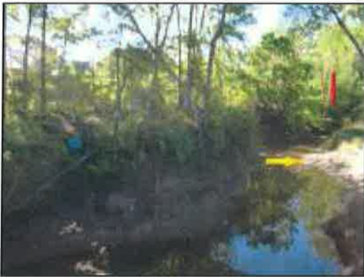
Figure 38: Looking upstream; the yellow arrow indicates the toe of a slope failure of the west bank; note the large leaning tree indicated by the red arrow.
