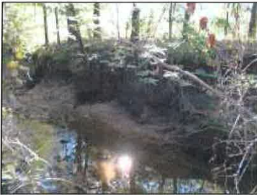
Figure 44: Looking downstream at east bank undercut by erosion
