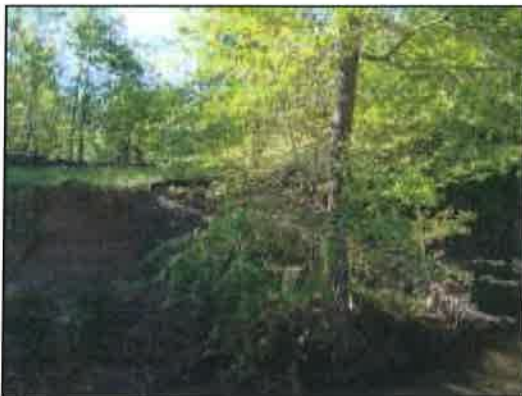
Figure 57: Outside bend erosion along a high bank on the east bank; note the tree that has re-rooted at the toe of the near vertical slope
