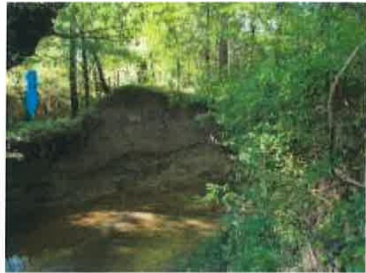
Figure 41: Bank erosion upstream of Leaning tree; the blue arrow is pointing to the flowline of the ditch beyond that serves as the outlet for the discharge from the pond in the adjacent subdivision
