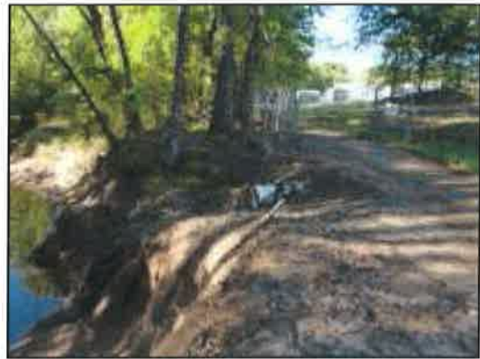
Figure 37: Second view of culvert crossing of access road; note how close to the top of the vertical bank is to the road
