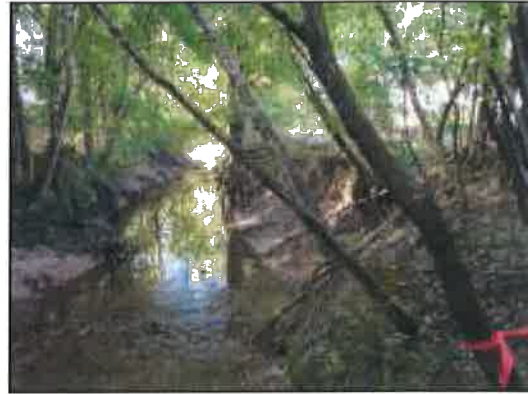
Figure 33: Looking upstream; note the sudden widening of the west bank where a bank failure has occurred and the more narrow section just upstream
