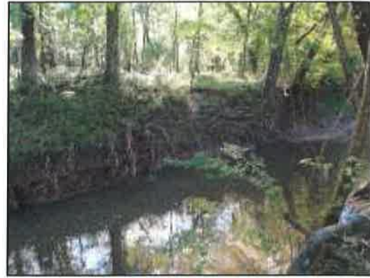
Figure 6: East bank just upstream of bank repair; note that root system of several trees are undermined
