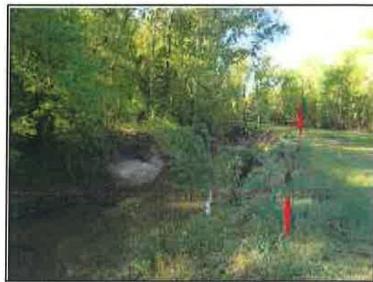
Figure 18: Red arrows indicate the ends of a vertical shear crack formed along the top bank
