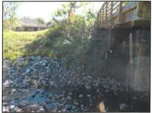
Figure 73: 2016 water line undermined and removed.
