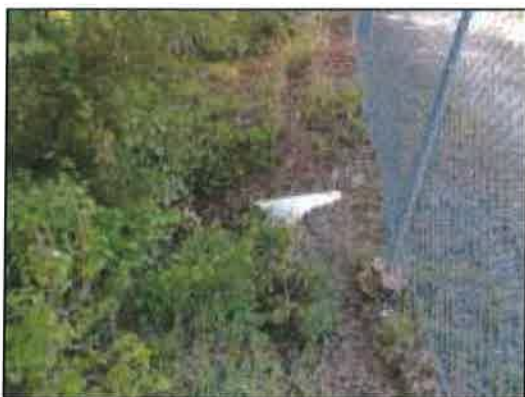
Figure 48: End of culvert from under gravel Drive; washout is overgrown.
