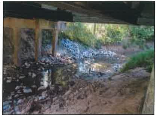
Figure 75: Approximately 1+ of additional pile length exposed in 2016
