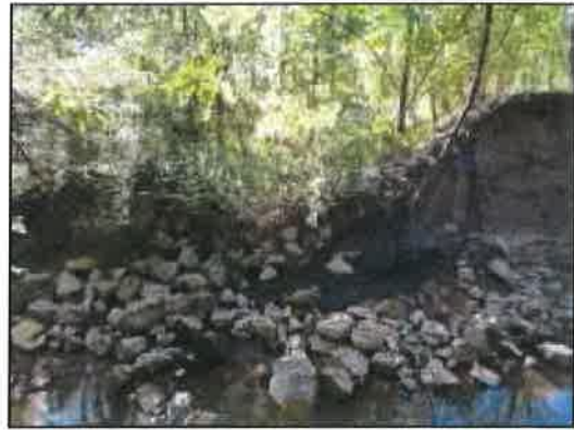
Figure 51: Looking up ditch serving as an outfall for part of the storm sewer system serving the adjacent subdivision
