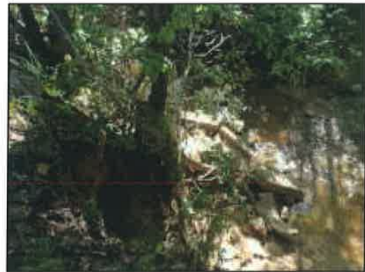
Figure 68: Broken concrete used as rip-rap at the upstream end of the failure shown in figure 67
