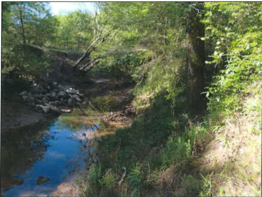
Figure 52: Looking upstream from same vantage point as figure 50; note the failure of the rip-rap at the end of the storm sewer outlet ditch, and the three trees that have slide into the stream channel
