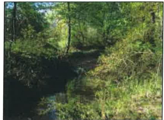
Figure 58: Just upstream of figure 57 looking upstream at bend erosion along a low bank on the east side
