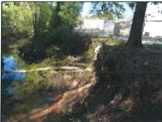
Figure 46: Closer view of slope failure shown in figure 45
