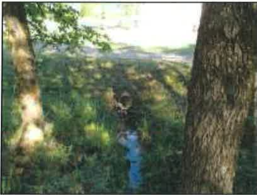
Figure 55: Outlet end of culvert from under gravel drive that discharges into the cantilevered pipe
