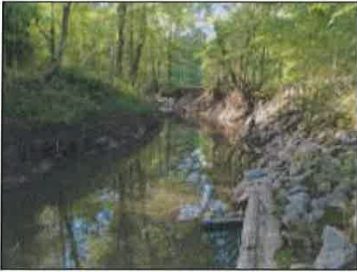
Figure 5: Stabilization of past bank failure; note the undermined and leaning trees just upstream of the bank repair
