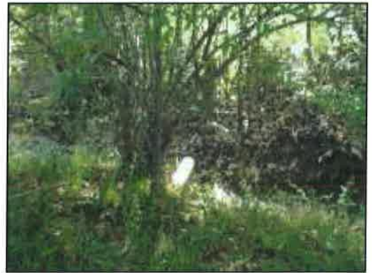
Figure 56: Pipe cantilevered from bank
