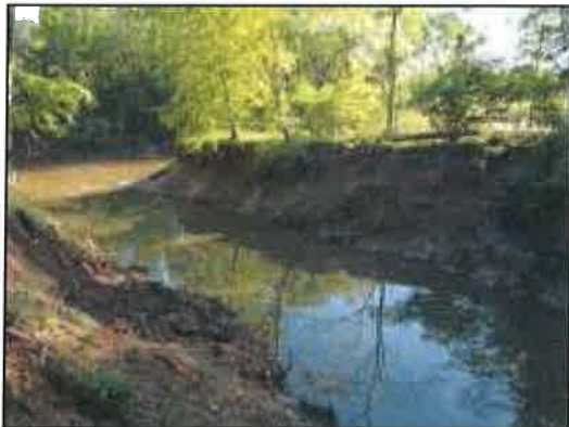
Figure 3: Evidence of recent bank erosion of the Lateral at the confluence
