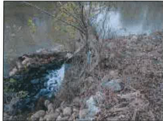
Figure 2: Sanitary Sewer Outfall into the Wolf River
