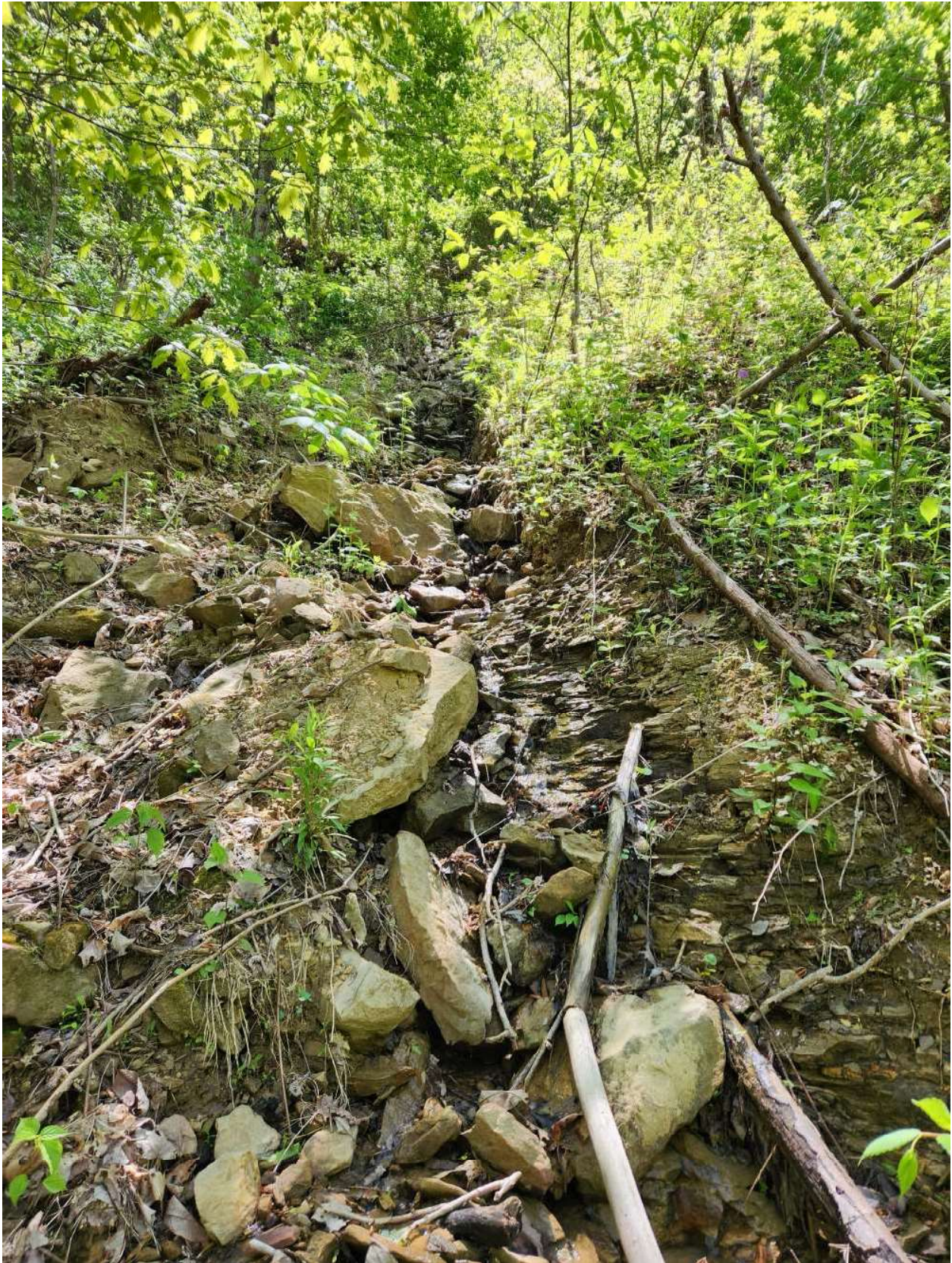
Location: 36.564896°, -83.840996° Date: 2023-05-04 Photograph #1 of channel 4A flowing over Pre-SMCRA highwall, taken by Phil Boggs viewing upstream or southeast.
